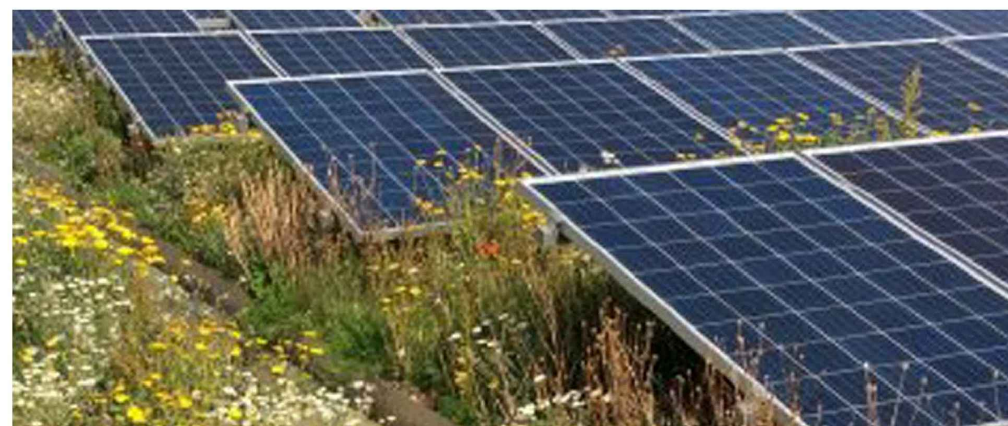
GREEN LIVING ROOF SYSTEM INTERDISPERSED WITH PV PANELS.
