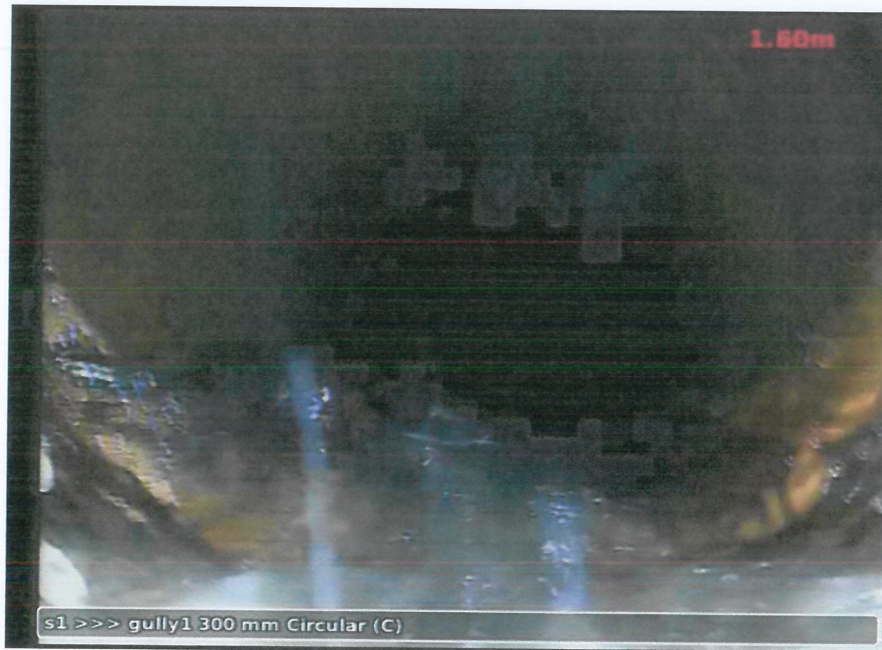
S1X_b5cbd597-4bfd-46ef-b02a-72fad86109fb_20210303_083646_549.jpg, 00:00:32, 1.71 m Roots, fine at joint
