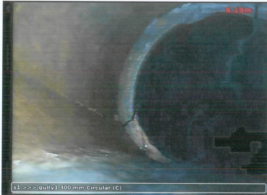
S1X_f6120a4c-e547-4d8c-bc76-be326122d481_20210303_083810_540.jpg, 00:00:49, 6.27 m Fractures, multiple from 9 o'clock to 3 o'clock
