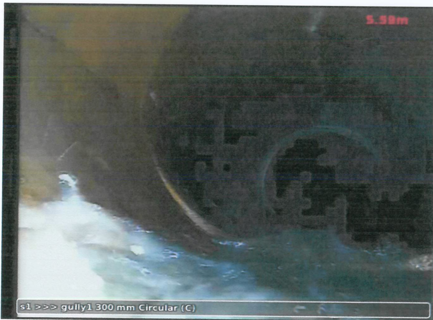
S1X_52854503-d1ea-4d91-8177-e7befb19290b_20210303_083723_541.jpg, 00:00:46, 5.59 m Fracture, circumferential from 9 o'clock to 12 o'clock
