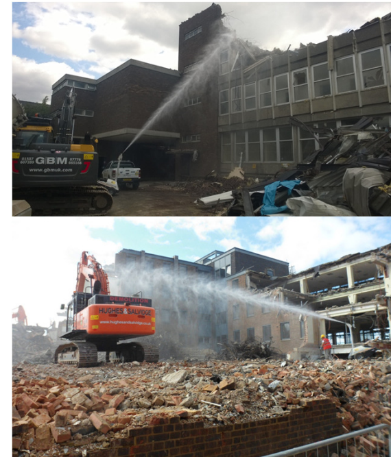
Water cannon dust suppression system
