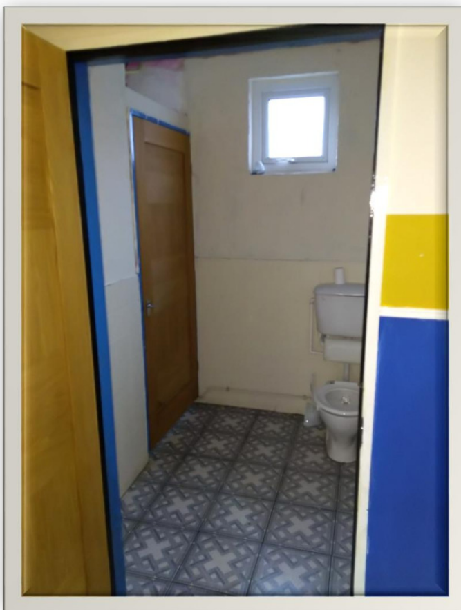
Left; Existing combined disabled and ladies toilet provision unacceptable with a toilet cubicle accessed via the current disabled toilet provision.
