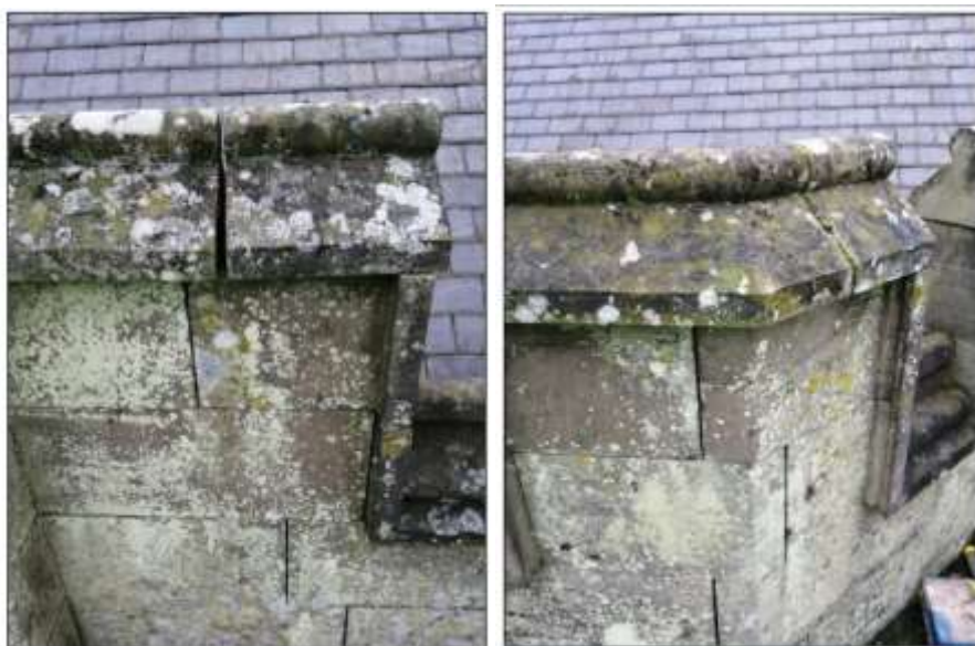
Photos of loose copings and crenellated parapet
