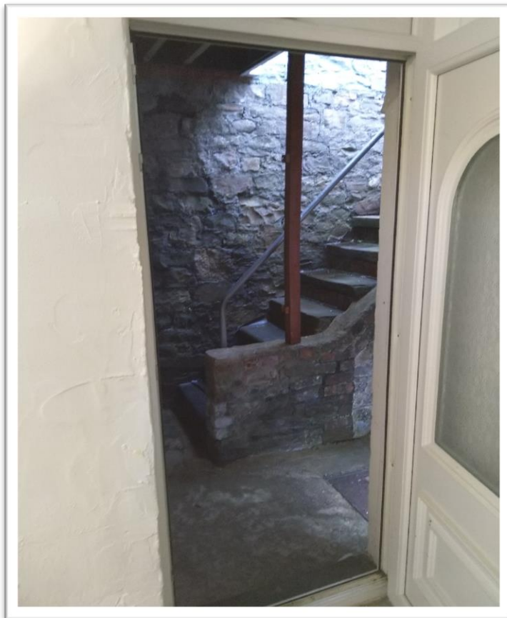
LEFT: Photograph looking out of the rear of the ground floor former retail space to the small rear passageway and steep external stone access stairs to the residential accommodation above. These stairs are steep, slippery when wet and difficult to negotiate despite the addition of the disability standard hand rail.
