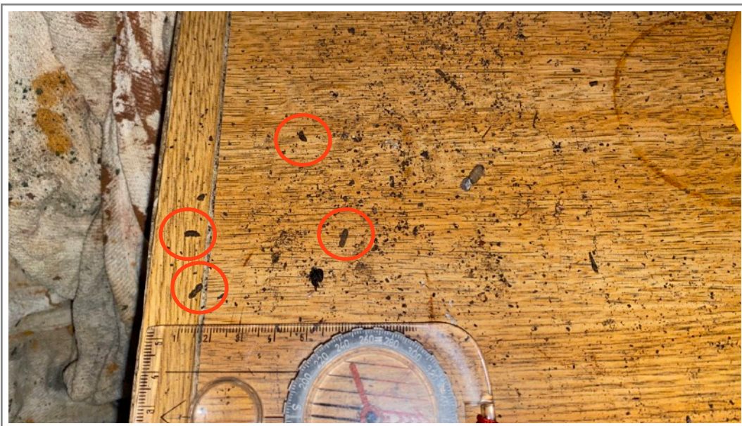
Photo 4: Guano inside garage (circled)
