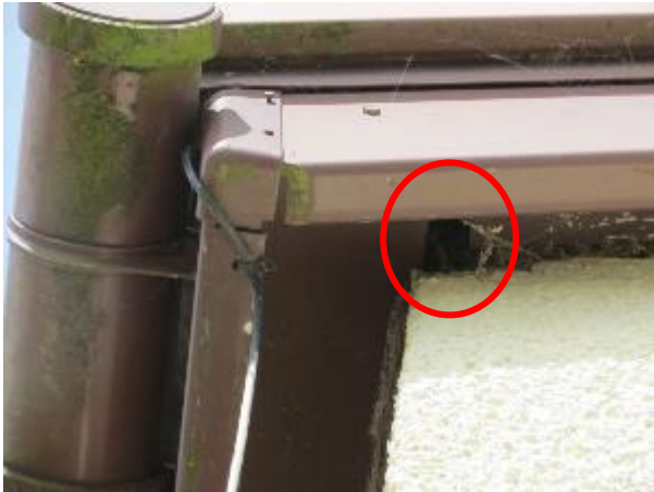
Photo 13: Hole in Soffit
