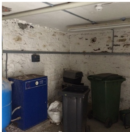
Figure 9. Boiler room in the basement.
