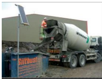
Figure 4: Washout into silt-buster
