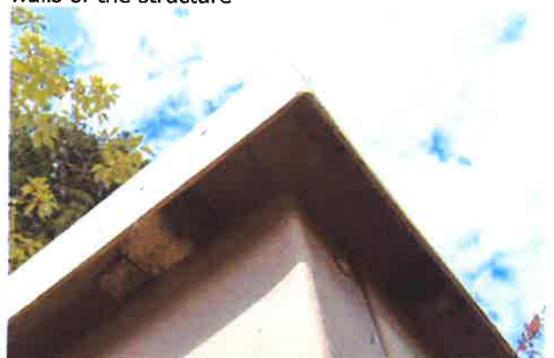
Photo 17: voids can be seen between the roof and walls of the structure
