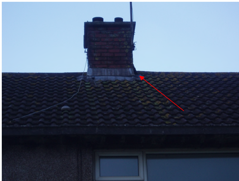
The loose flashing found on two of the chimneys (indicated by arrow)
