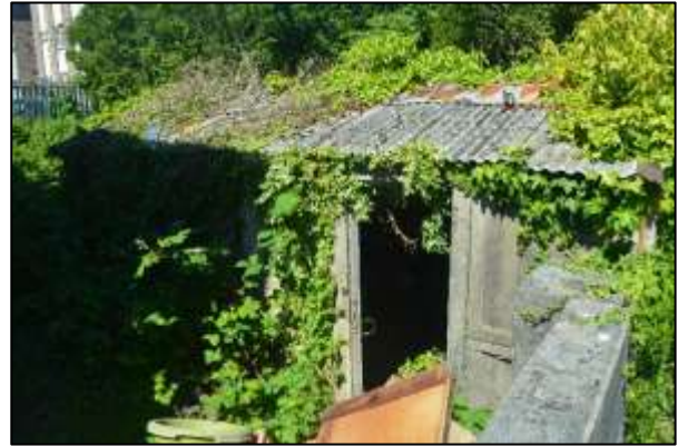
Photograph 10 – Small garden shed constructed of asbestos type material and corrugated metal, taken from garden wall.
