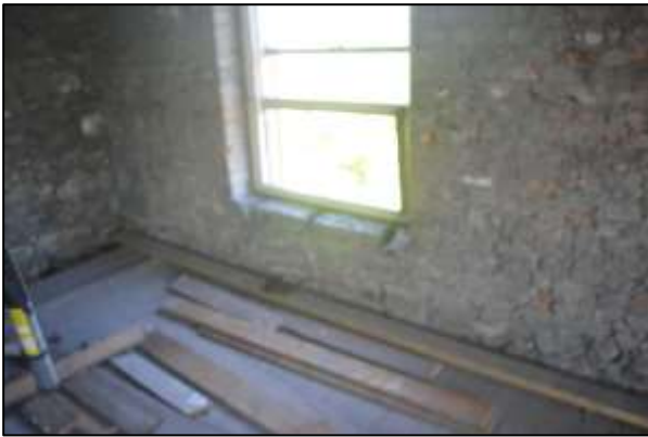
Photograph 3 – First floor window on northern elevation, access point to the inside of the building as it has been left open.
