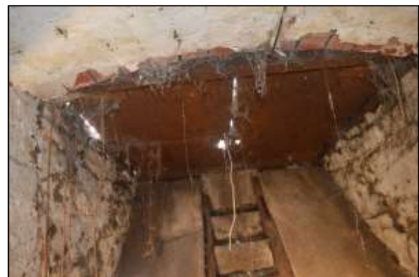
Photograph 6 – Cellar hatch, taken from inside the cellar. Showing access points to cellar in the form of gaps around the hatch.
