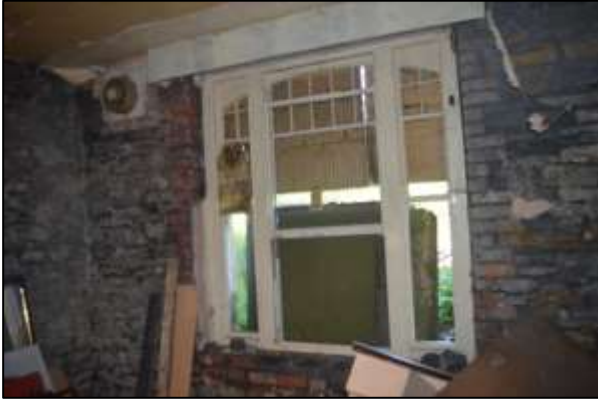
Photograph 7 – Ground floor window on northern side of the building. Access point to the interior as it has missing panes.
