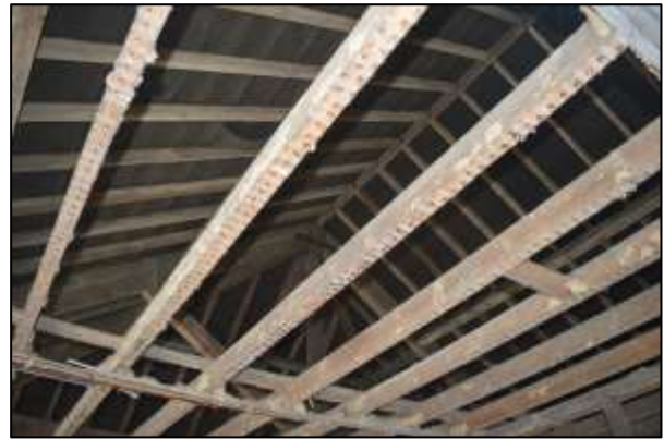
Photograph 4 – interior view of the roof, with ceiling missing, taken from the first floor.
