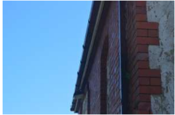
Photograph 8 – Soffit boarding on the northern elevation, with gaps present beneath.
