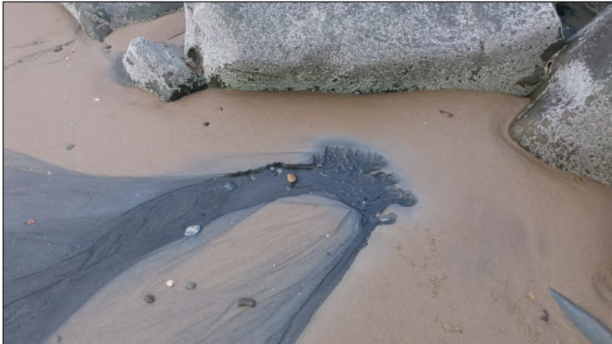
Photo shows discharge of visually contaminated water from the base of the sea wall (SW1)
