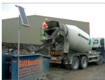
Figure 6: Washout into silt-buster
