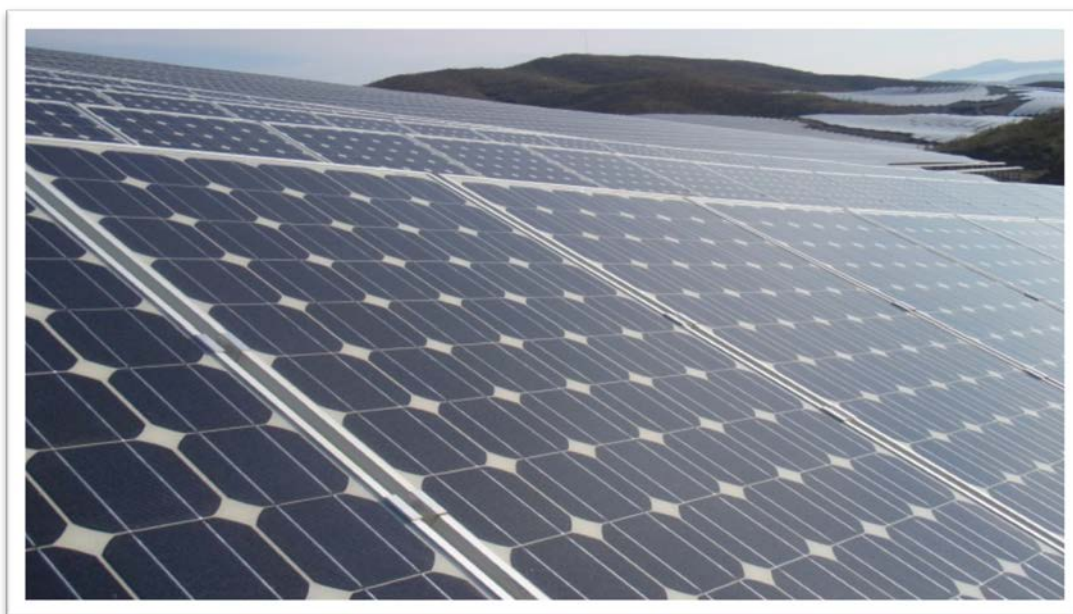
Plate 1: Typical Solar Panel
