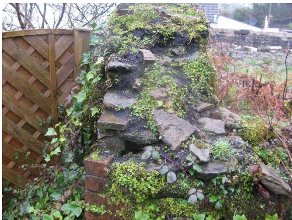
Internal void within stone-wall on the south-west site boundary.
