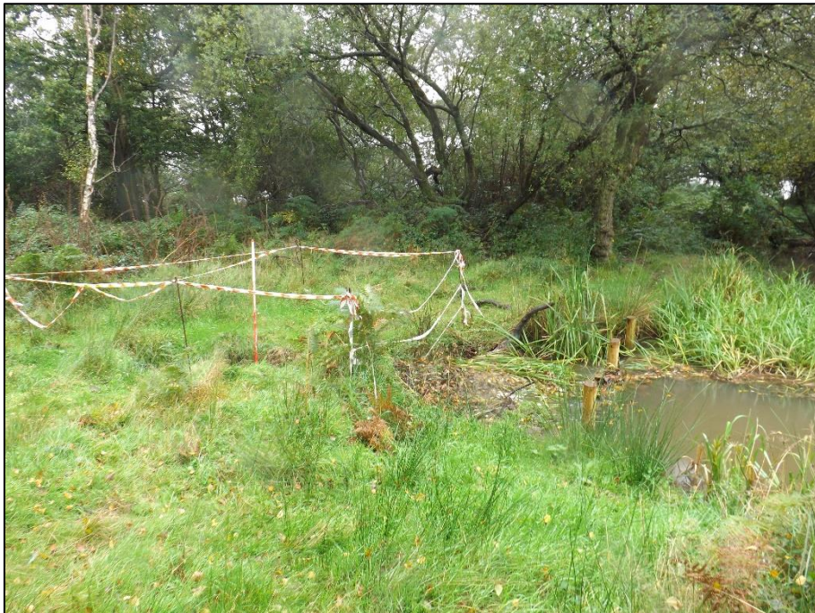
Plate 6. General view of clogged Structure 2. View to west. Scale just visible within the red and white taped area is 1m.
