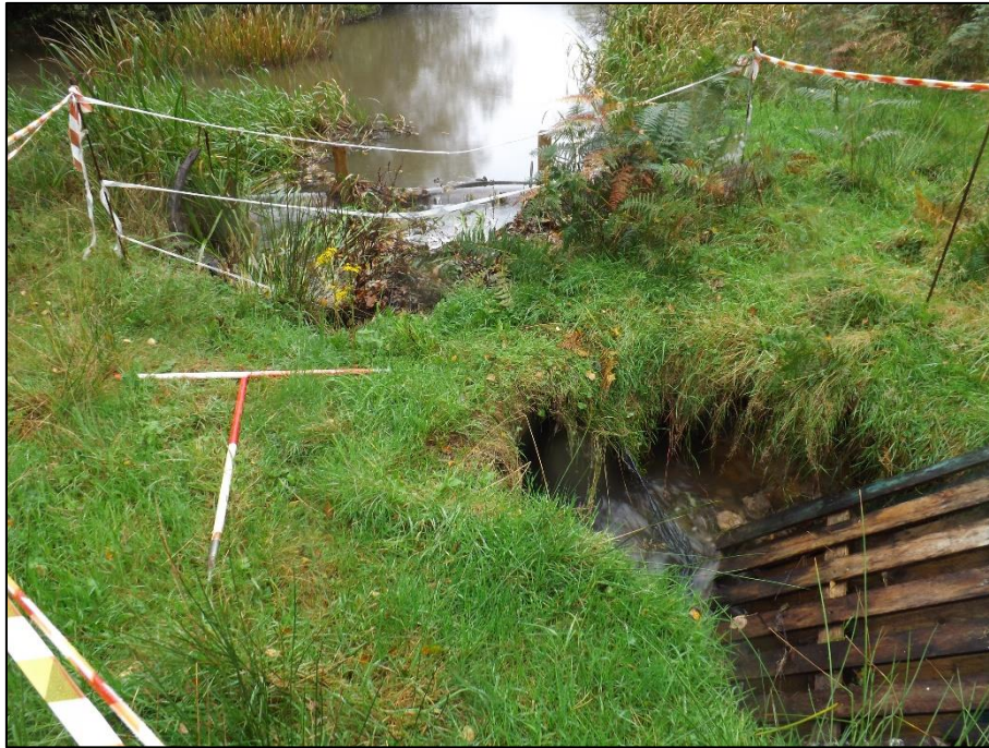
Plate 8. Area of subsidence immediately south of the water inlet of Structure 2. View to north, scale divisions 0.5m.
