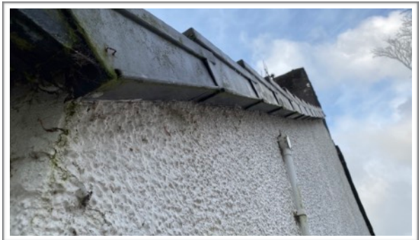
Photo 2: West facing wall/soffit interface
