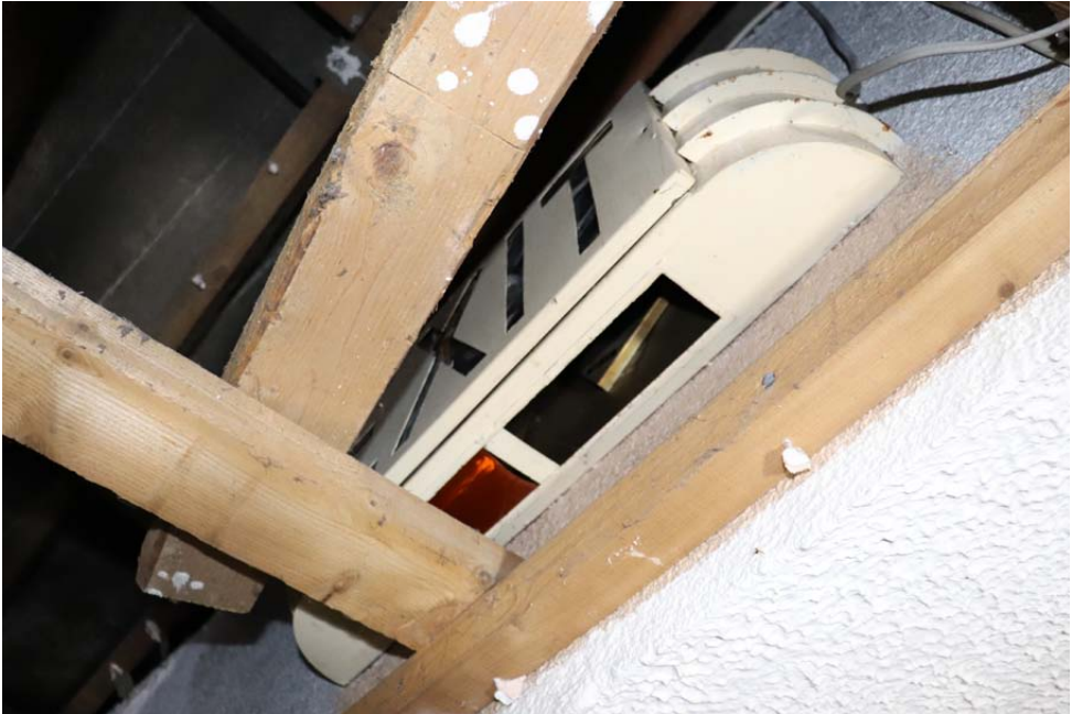
View of Art Deco style 'emergency escape' internally lit sign
