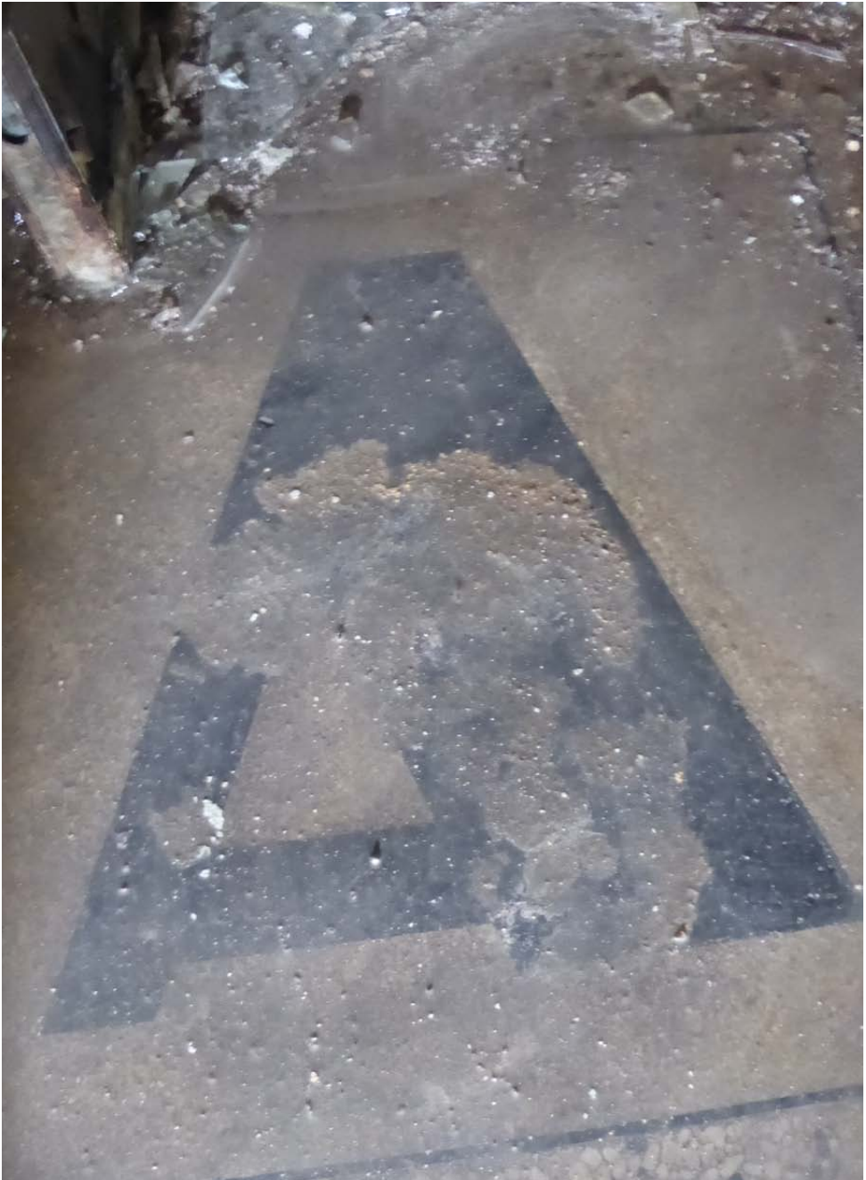
View of the final 'A' of the 'PLAZA' floor lettering which is damaged
