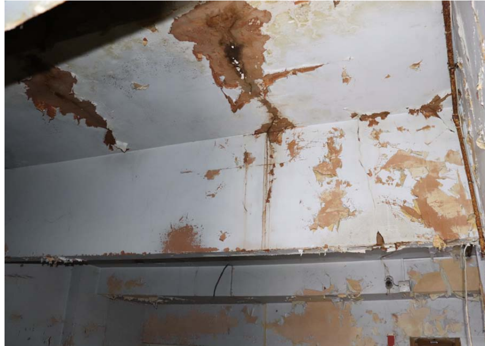
View of the concrete soffit with spalling concrete & damaged re-bar
