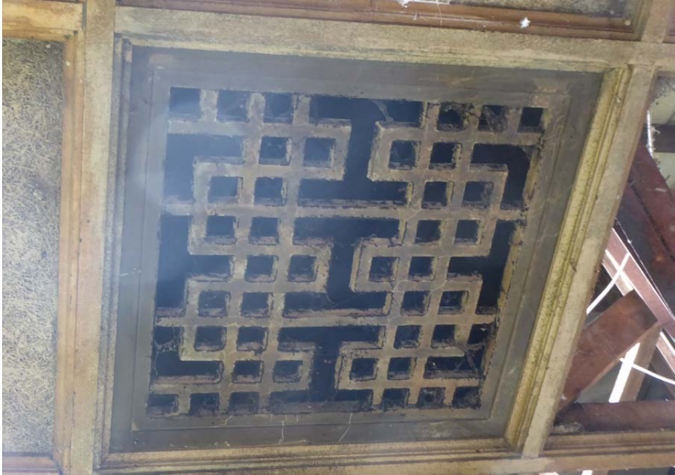
View of ventilation grille within ceiling
