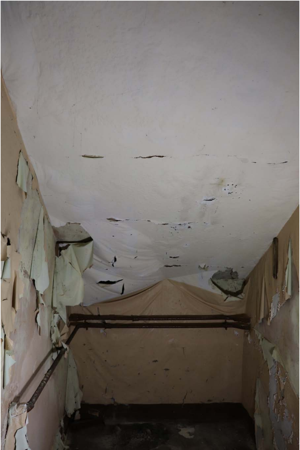
Peeling Paint & Plaster to Walls & Ceiling, which is sloping soffit
