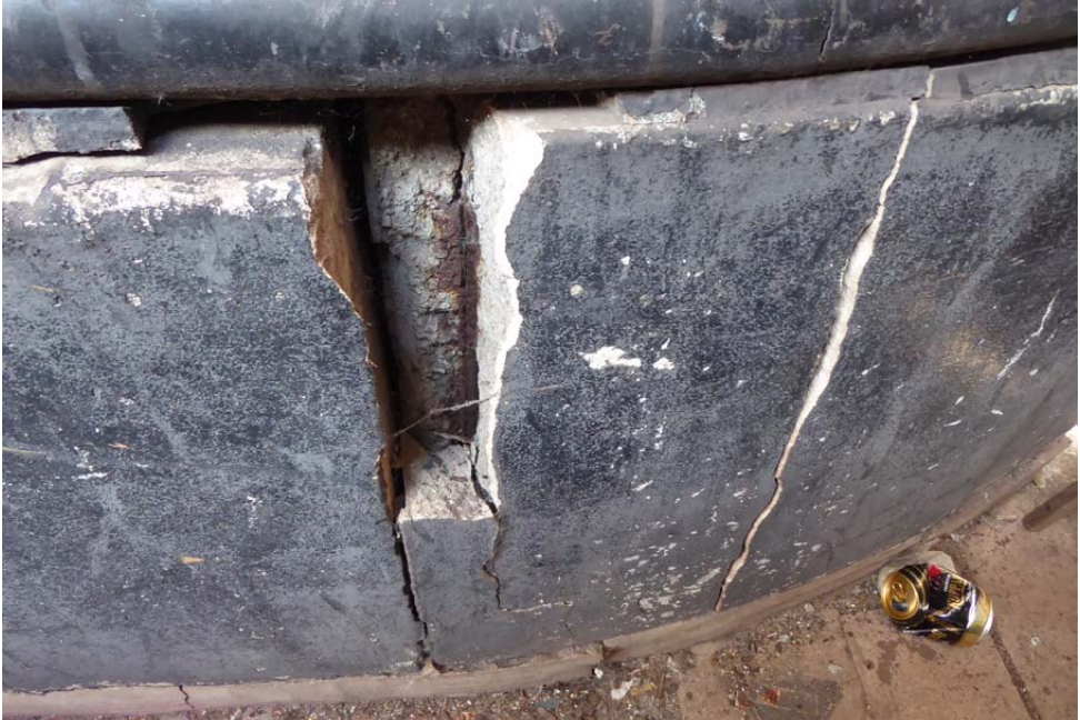
N Example of Damage to Masonry
