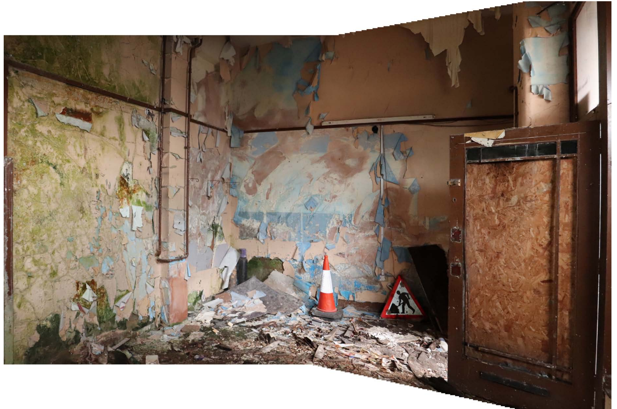
View east end of Retail space, with external door to right, showing painted plastered walls in poor condition
