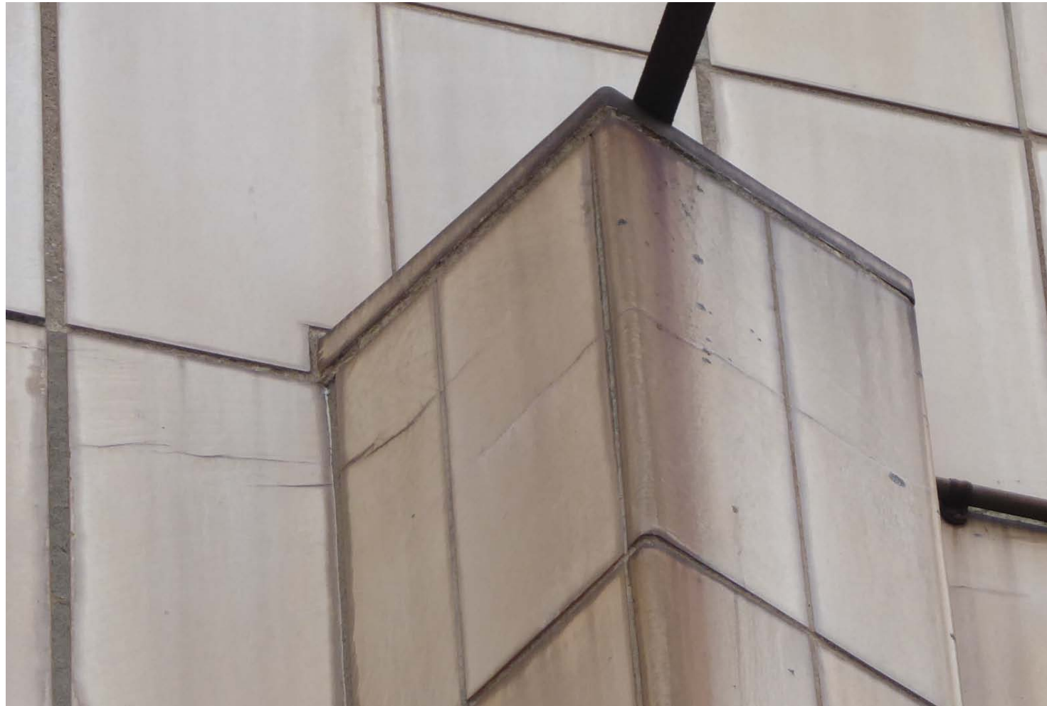
View of a crack running through a series of faience tiles on the top of one of the lighting columns
