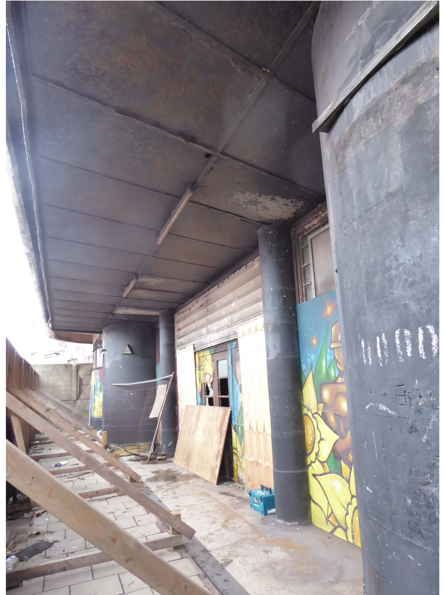
View of the bank of main entrance boarded up with the metal canopy overhead
