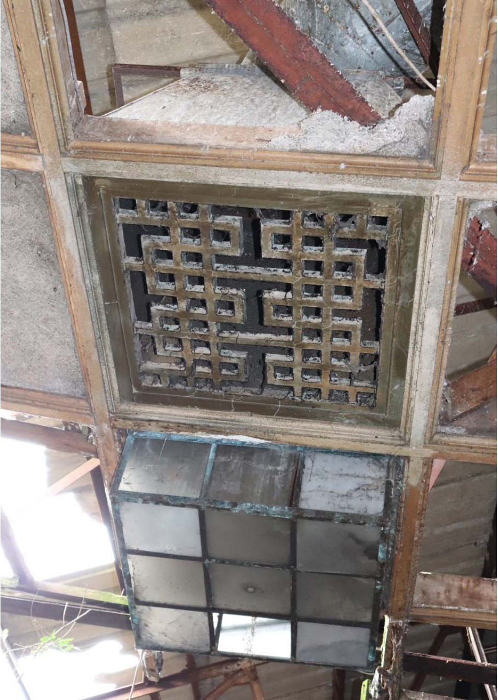
View of ventilation grille and light within ceiling
