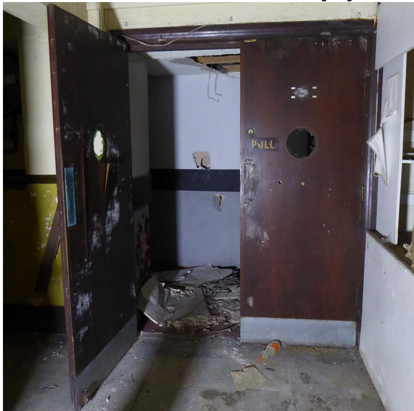
View of one set of doors - to the west cinema - which is in a reasonable condition
