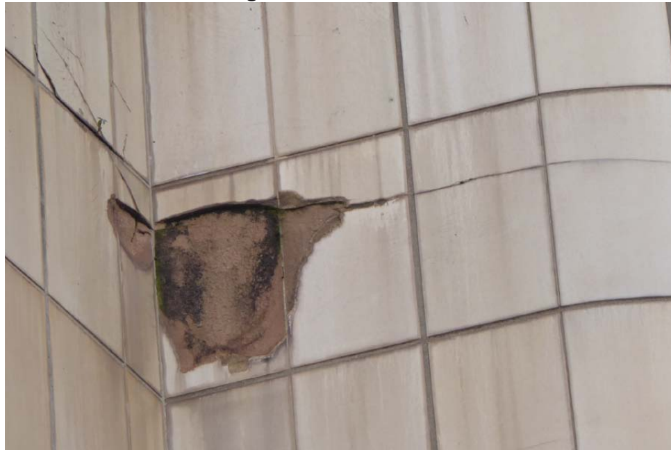
B Faience Tiling probably needing replacement
