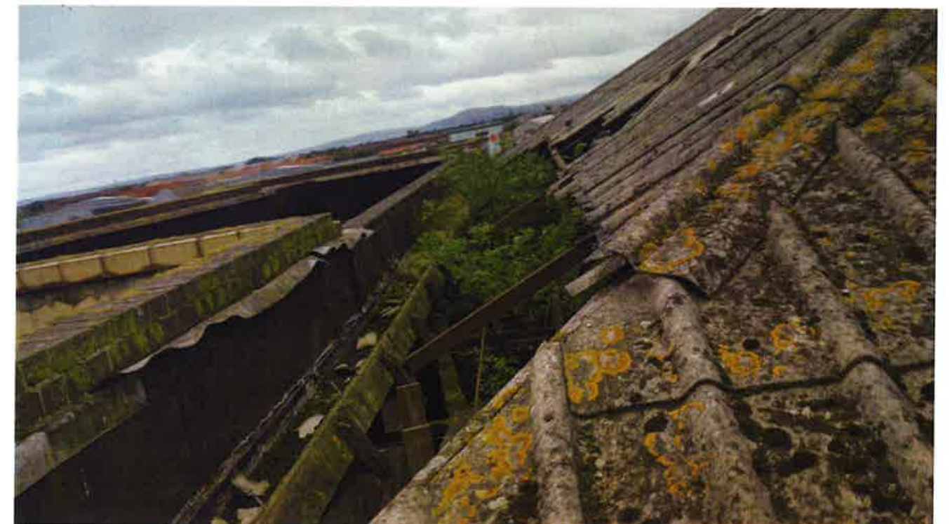
Broken section of asbestos cement roof sheeting, exposed steel trusses (rusted) to the elements (Photograph taken from MEWP July 2017)
