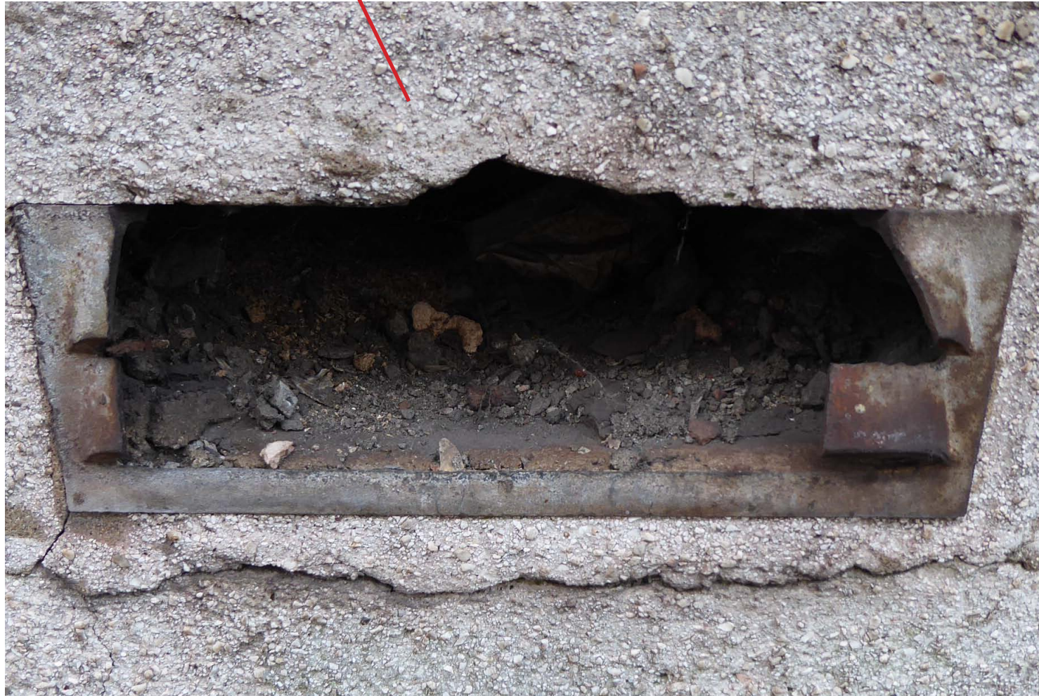
View of one of the broken low vents to the auditorium and cinema
