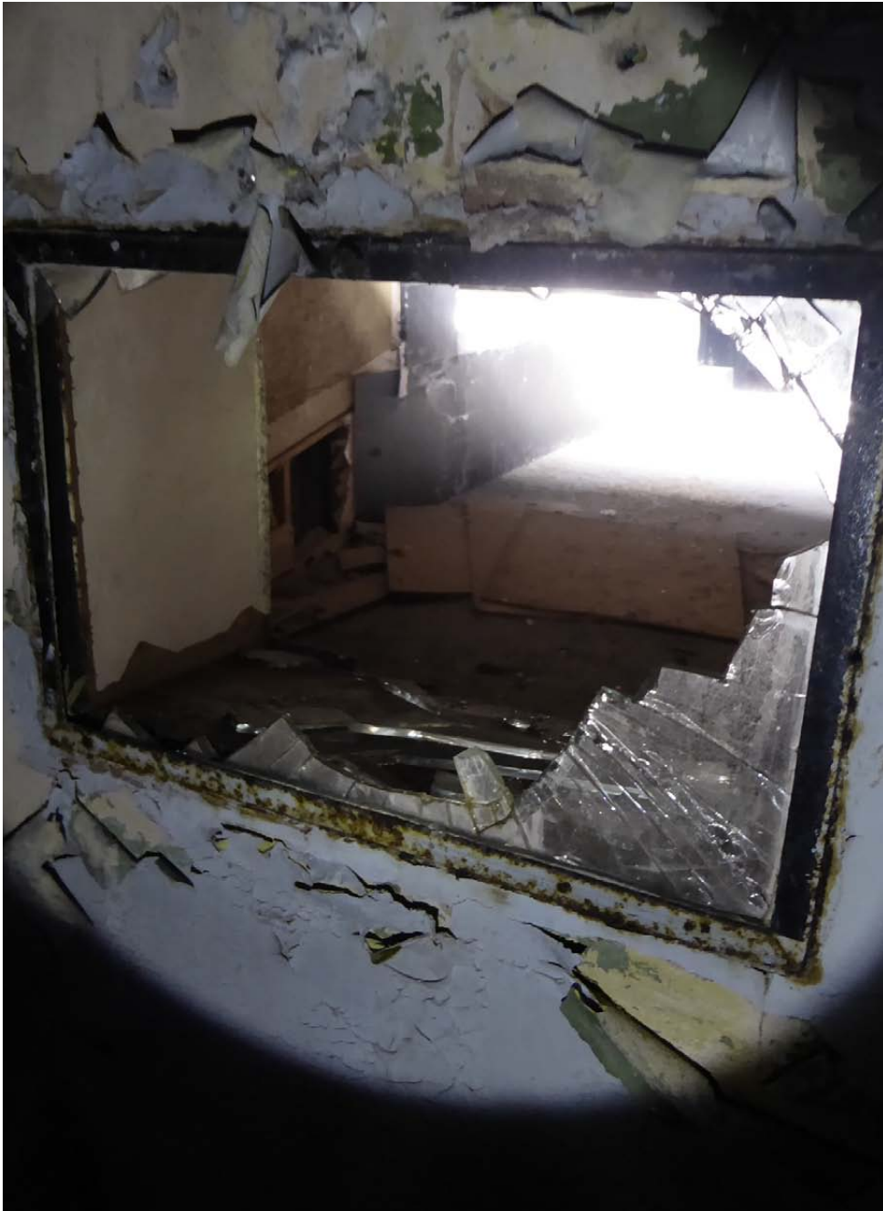
View of one of the projection window with the broken glass
