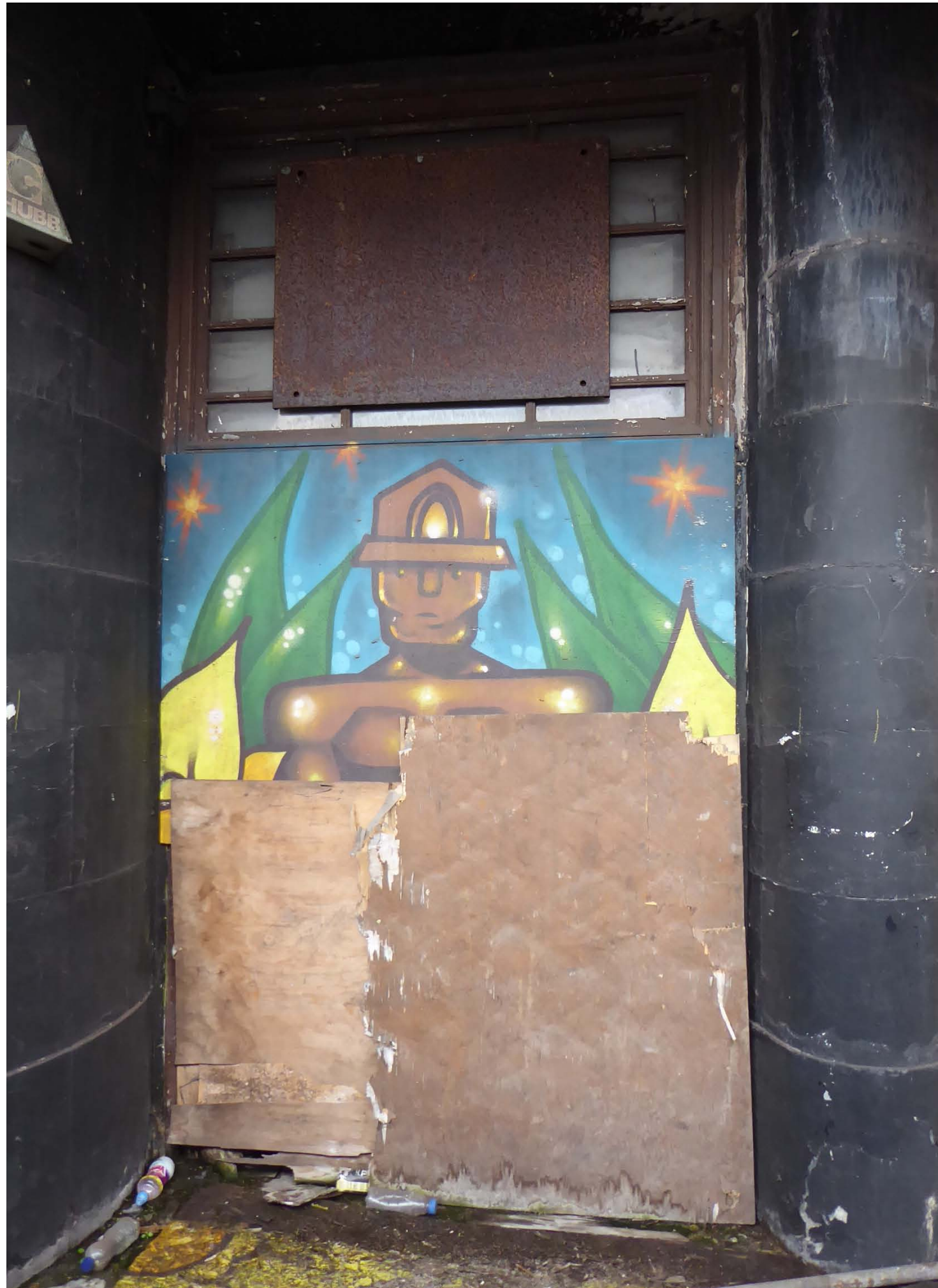
View of boarded up left hand large timber-frame glazed screen to side of bank of entrance doors
