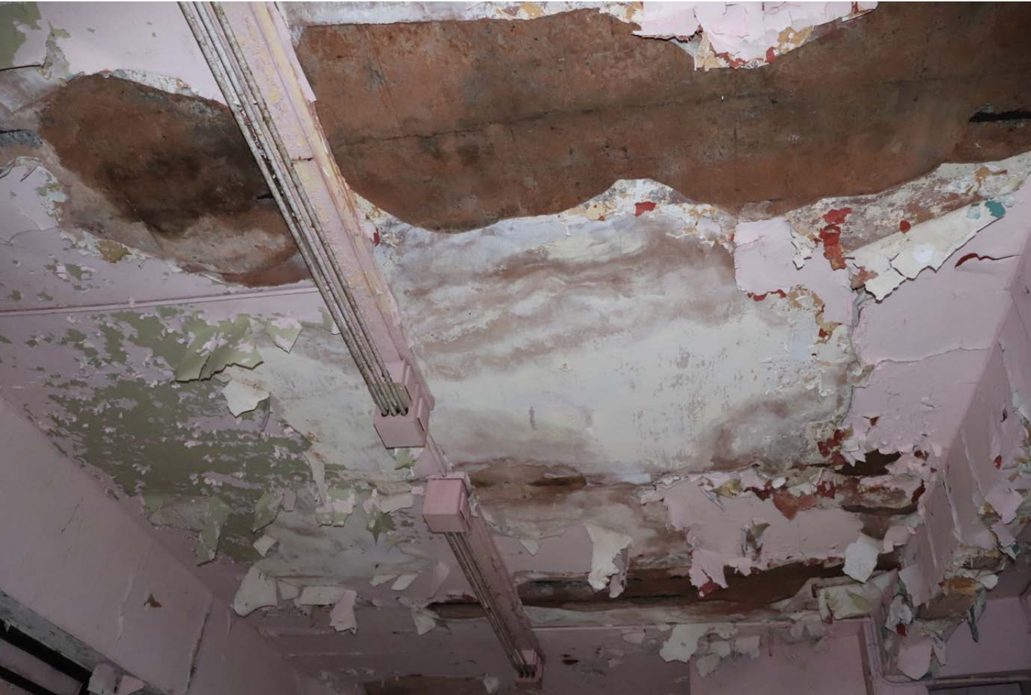
View peeling Paint, damaged Plaster and damaged Concrete Soffit to Ceiling
