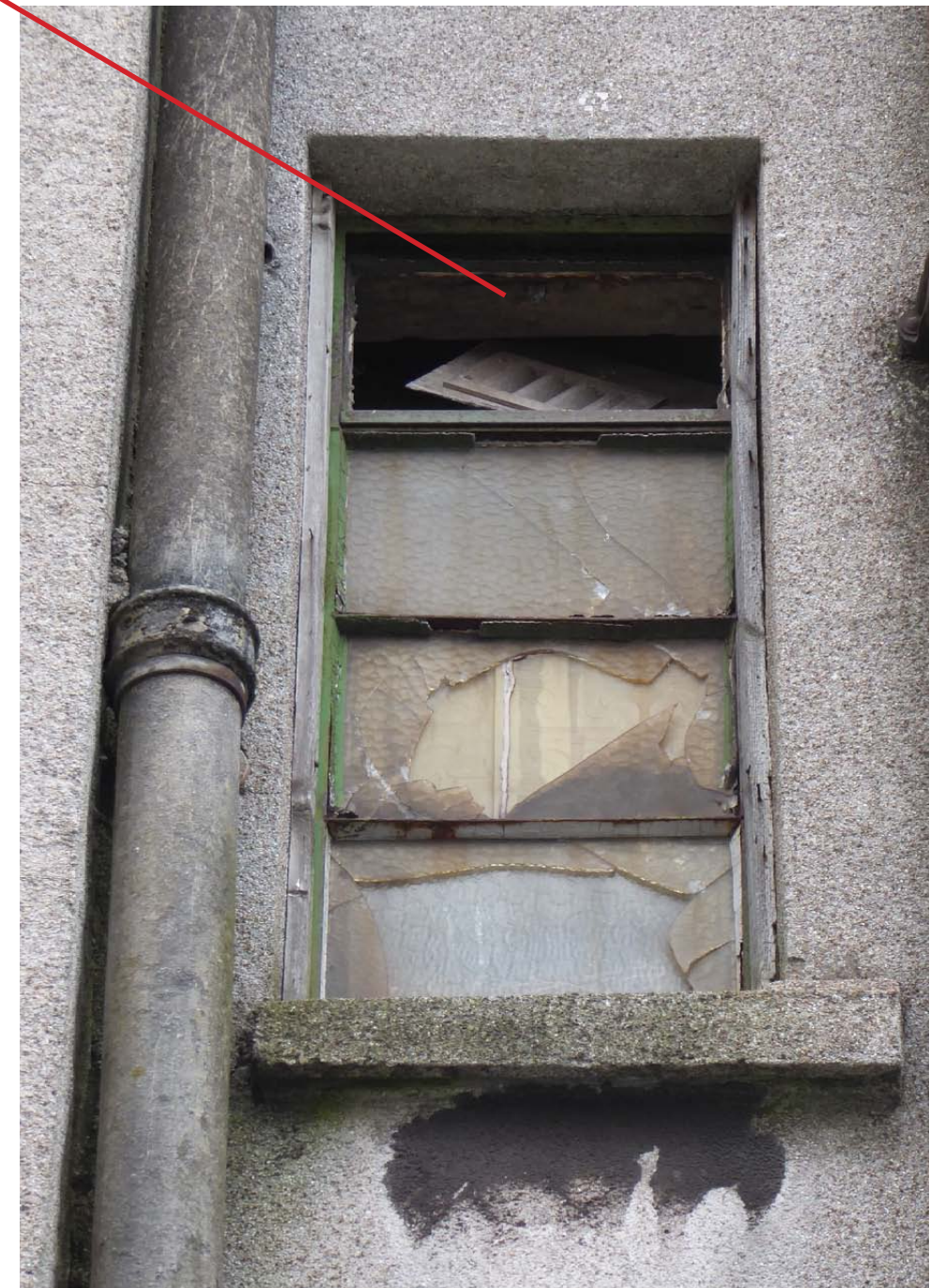
View to damaged window to first floor toilet
