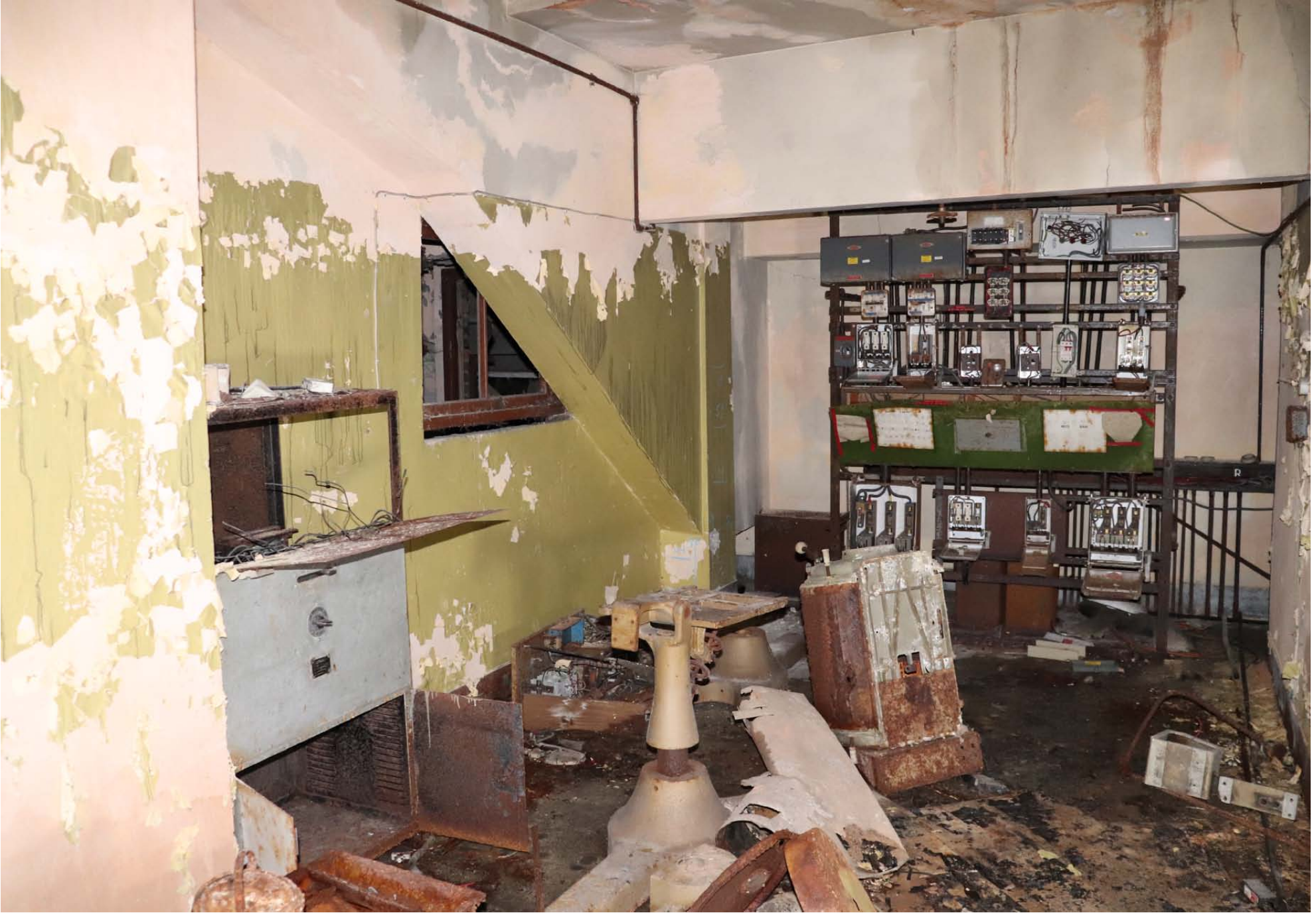
View of room from entrance door with switch gear at end
