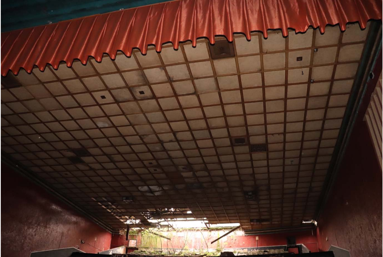
View of ceiling to Auditorium as seen from forestage with hole of roof at far end
