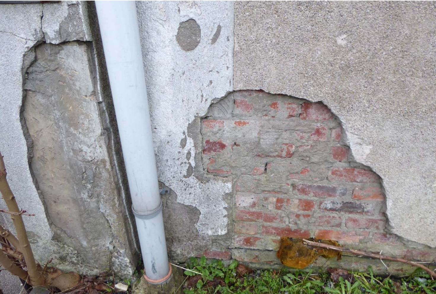
View of damaged render to the rear elevation showing the concrete frame and brick infill
