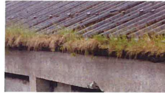
Close up of overgrowth (June 2017)
