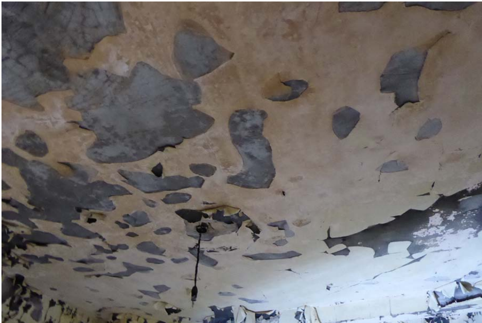
View of peeling paintwork to plastered concrete soffit
