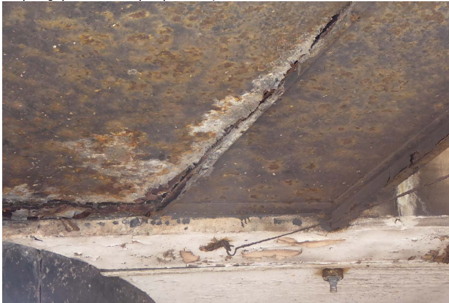
This photograph show how badly the panels and frame have been corroded
