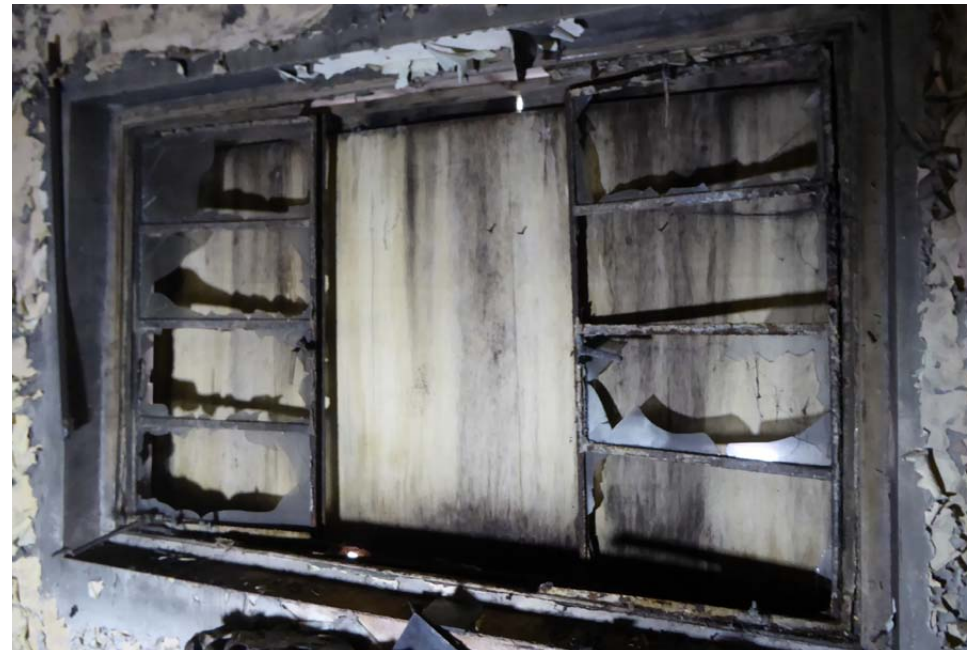
D Crittall Window to be Replaced like-for-like - Window F8
