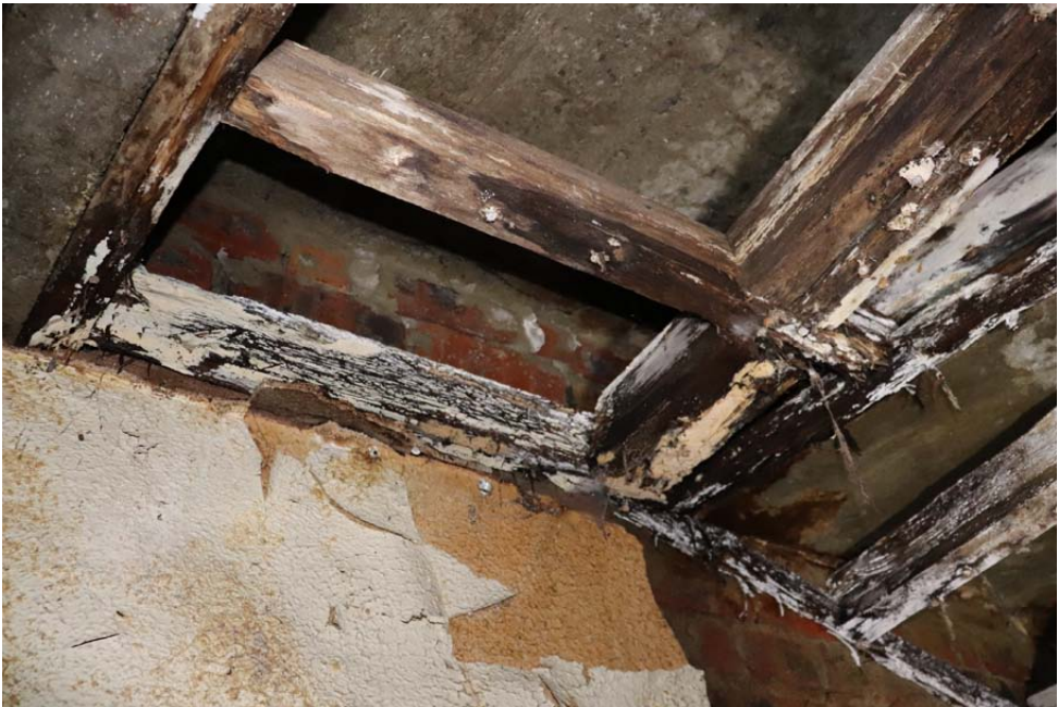
View of rot spores caking timber to underside of stairs
