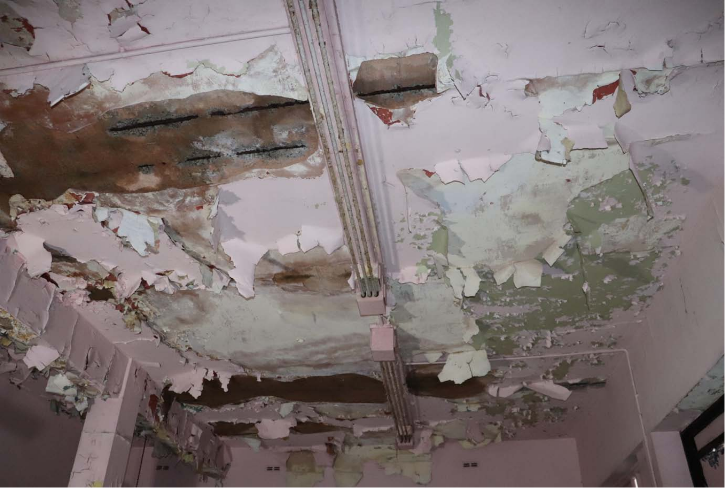
View peeling Paint, damaged Plaster & damaged Concrete Soffit to Ceiling with exposed Reinforcement
