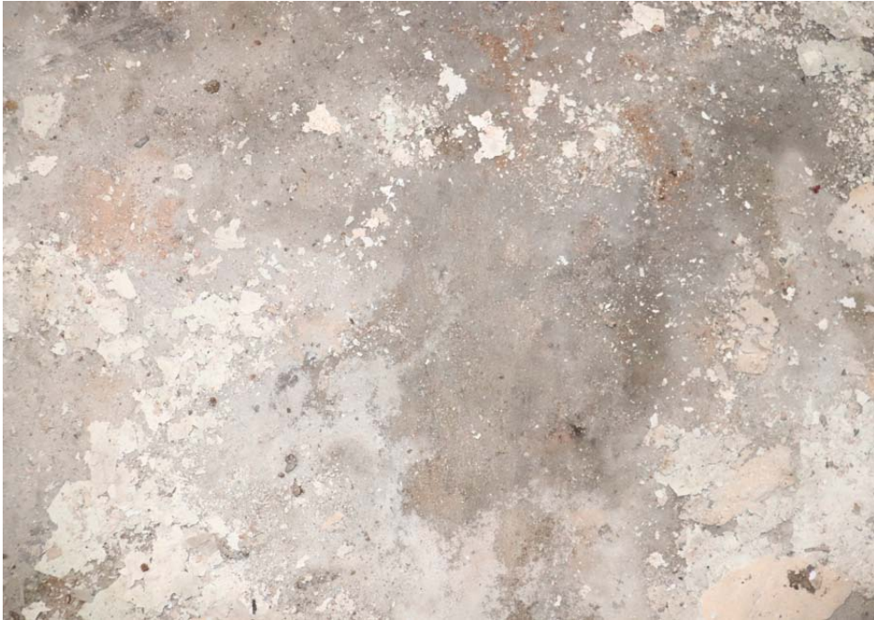
Flaking Paintwork to Concrete Floor
