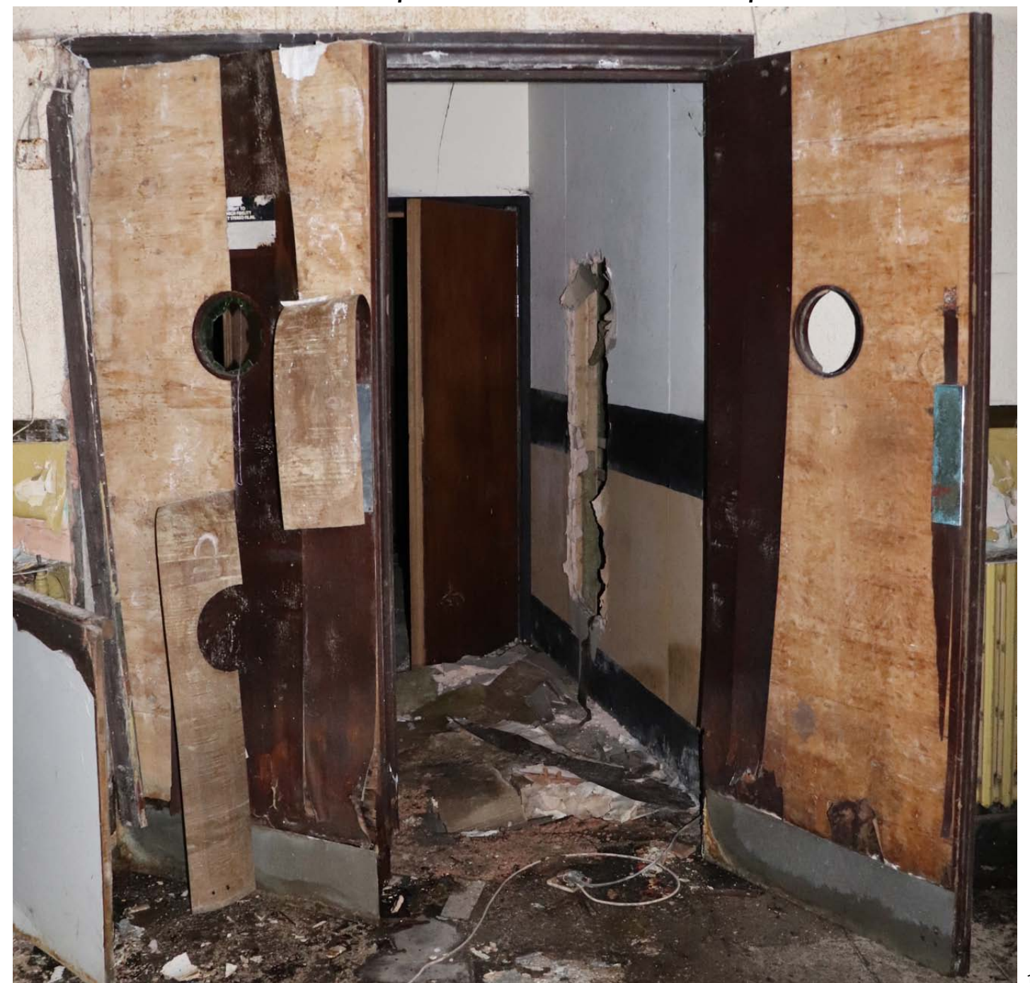
View of one set of doors - to the central corridor to the auditorium - which is in a very poor condition
