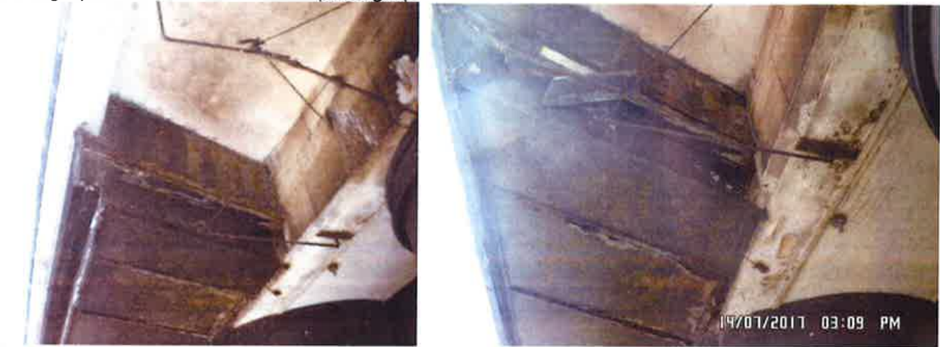
Corroded metal soffit panels (2012)
