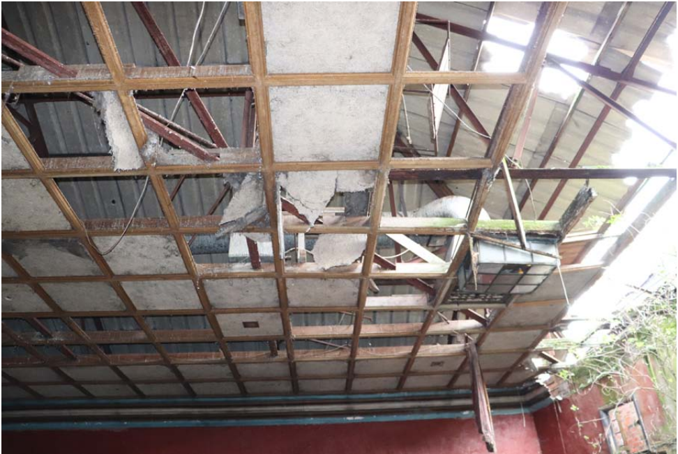
View of the ceiling looking eastwards with the large hole to the right
