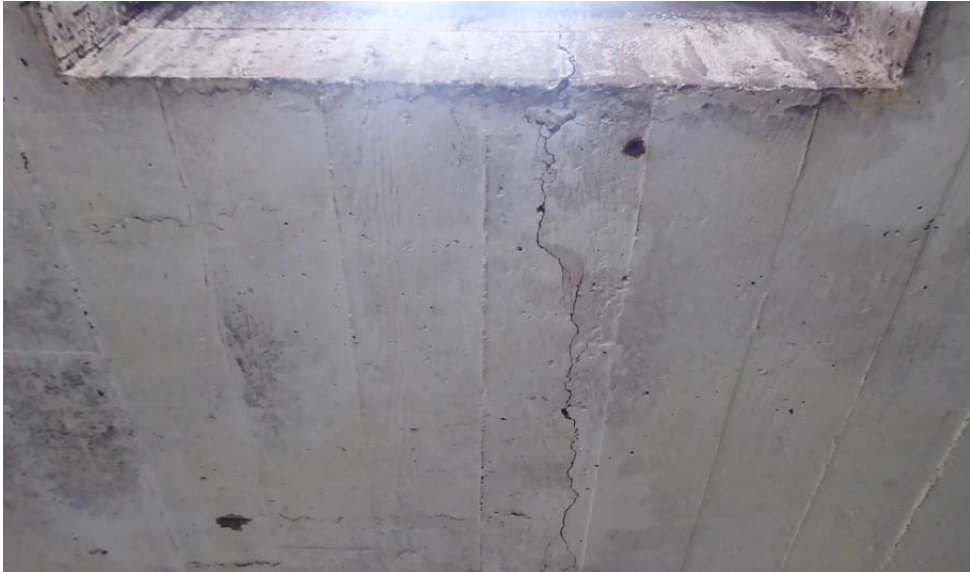
View of opening in soffit with start of long crack
