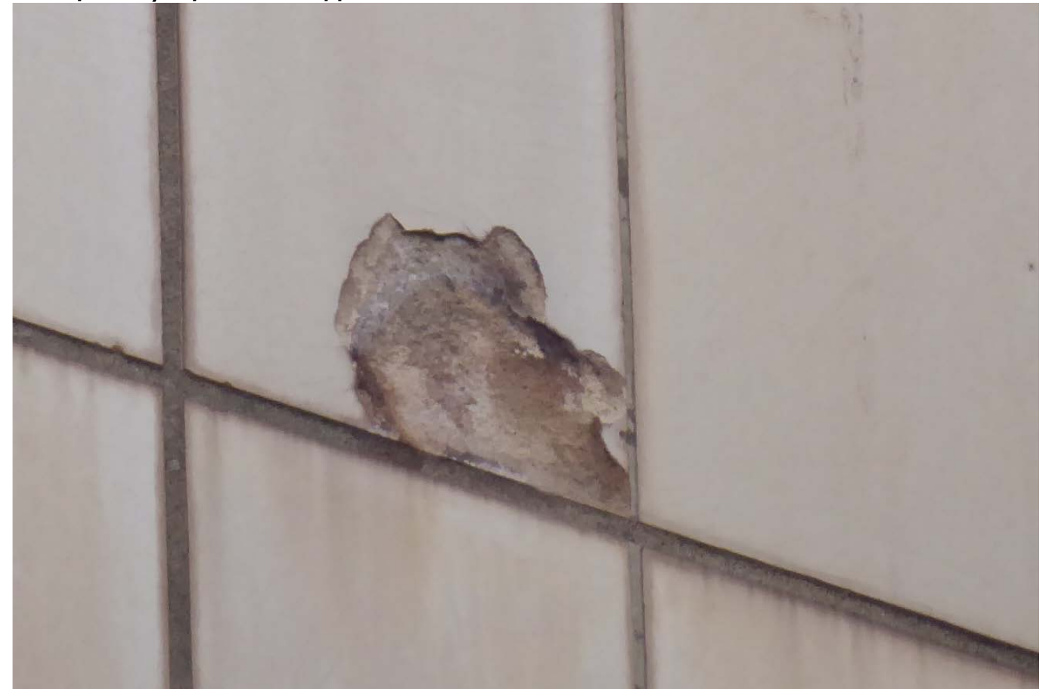
View of a badly defaced faience tile
