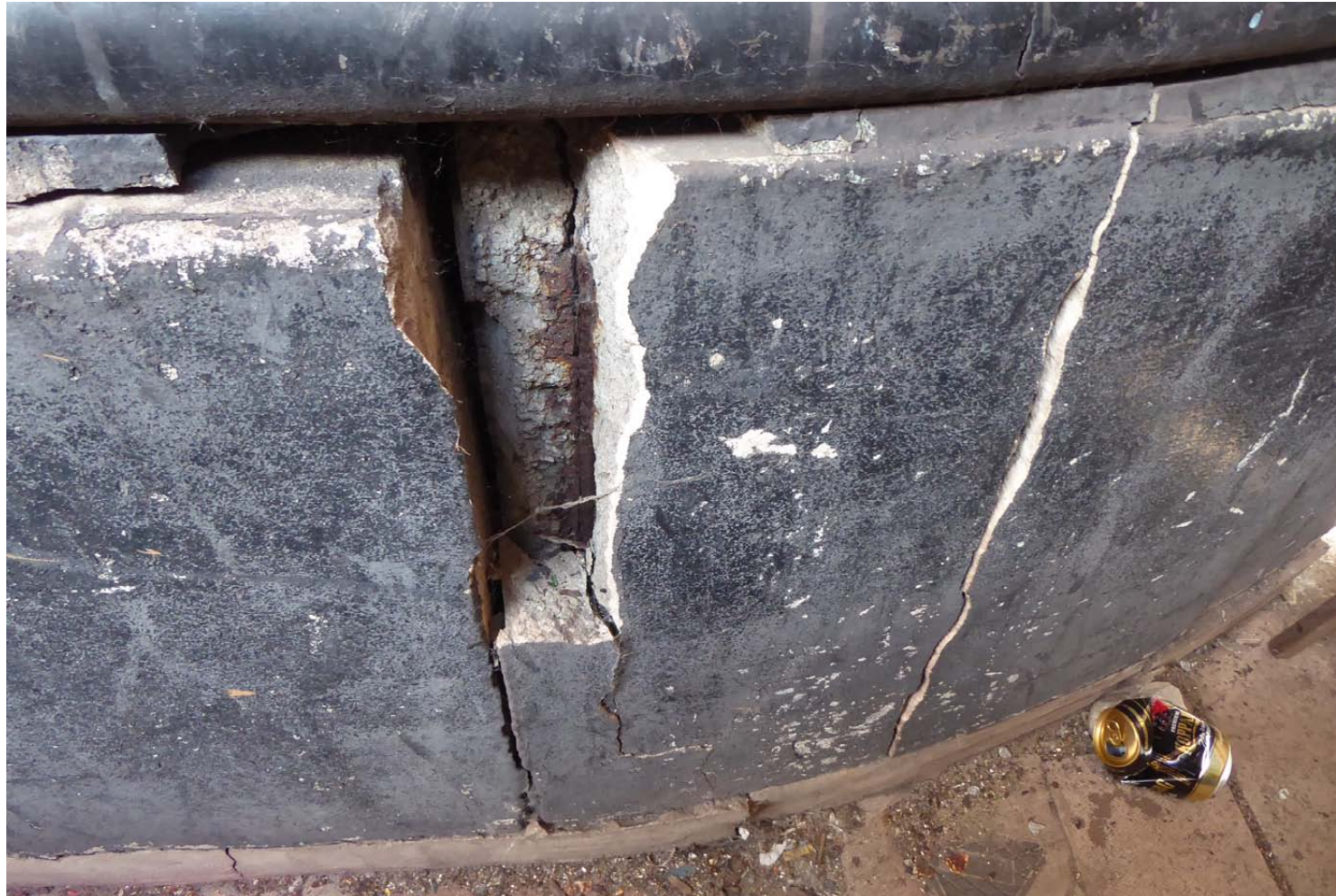
View of spalled surface to plinth showing corroded steel behind which presumably caused the spalling
