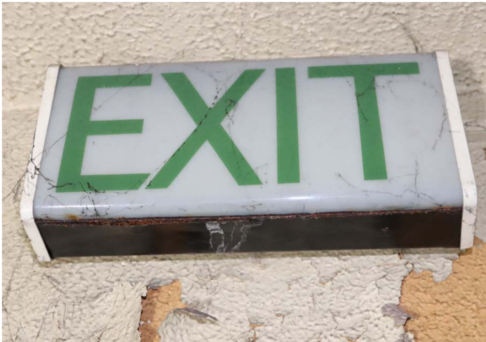
View of illuminated exit sign at the rear of the space
