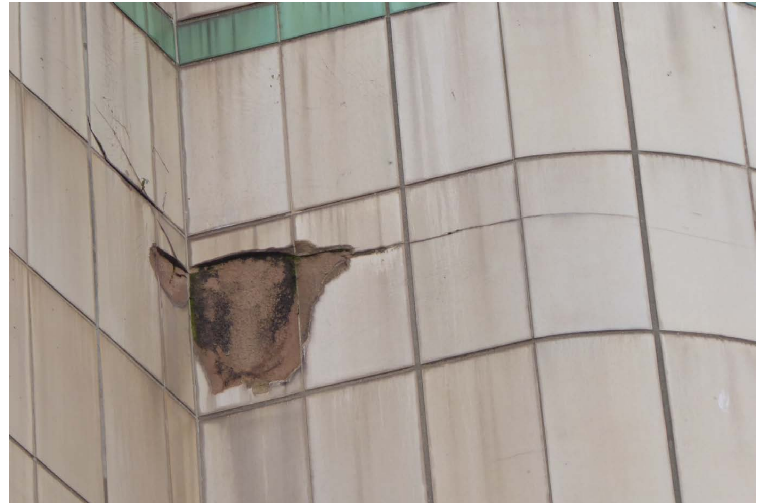
View of a badly defaced series of faience tiles
