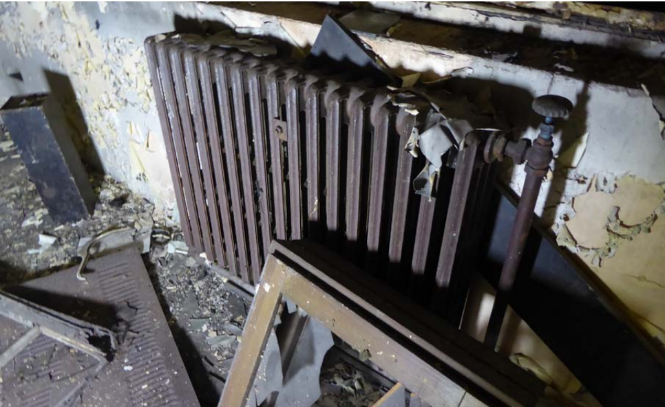
View of cast iron radiator in space
