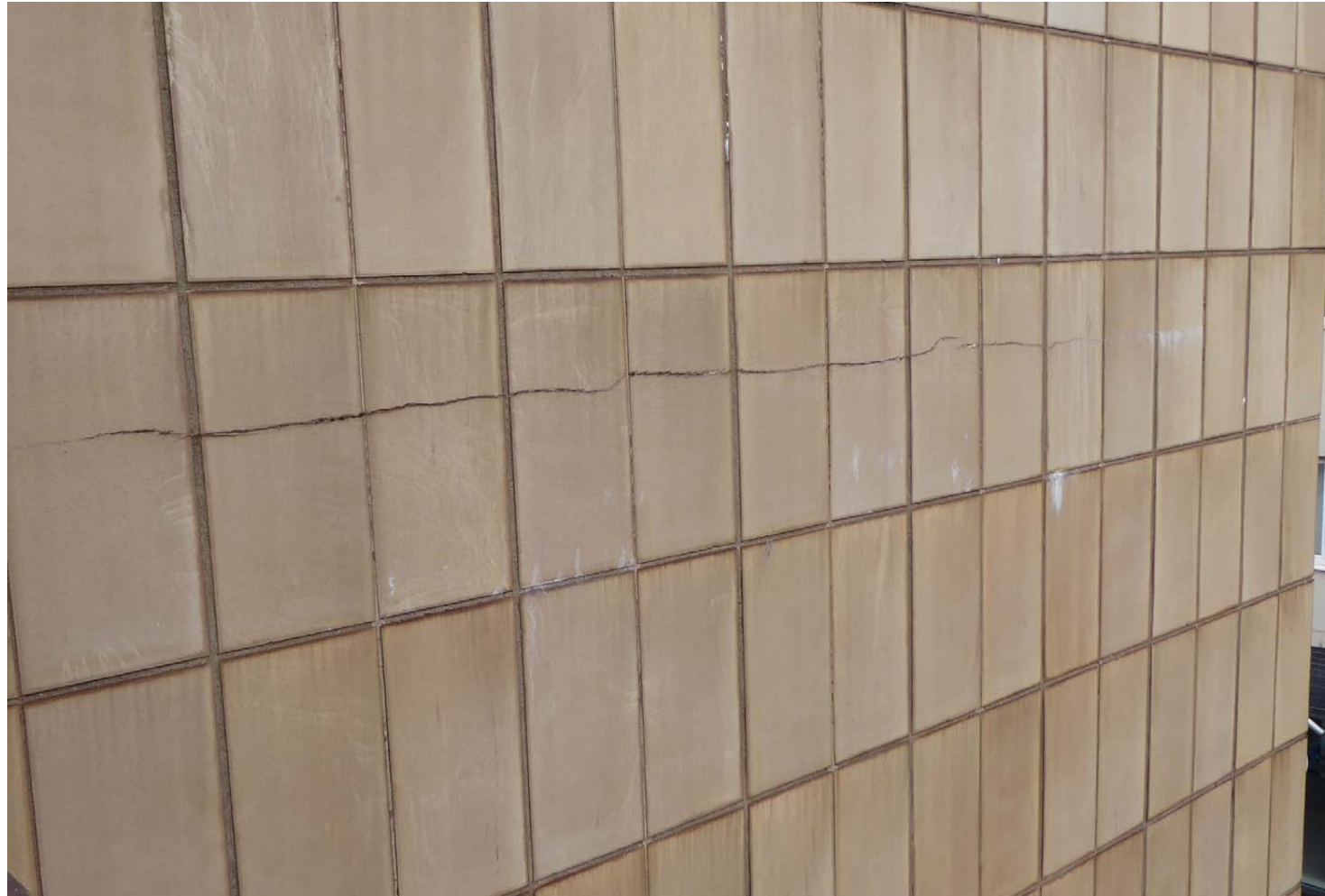
View of one of the cracks running through a series of faience tiles
