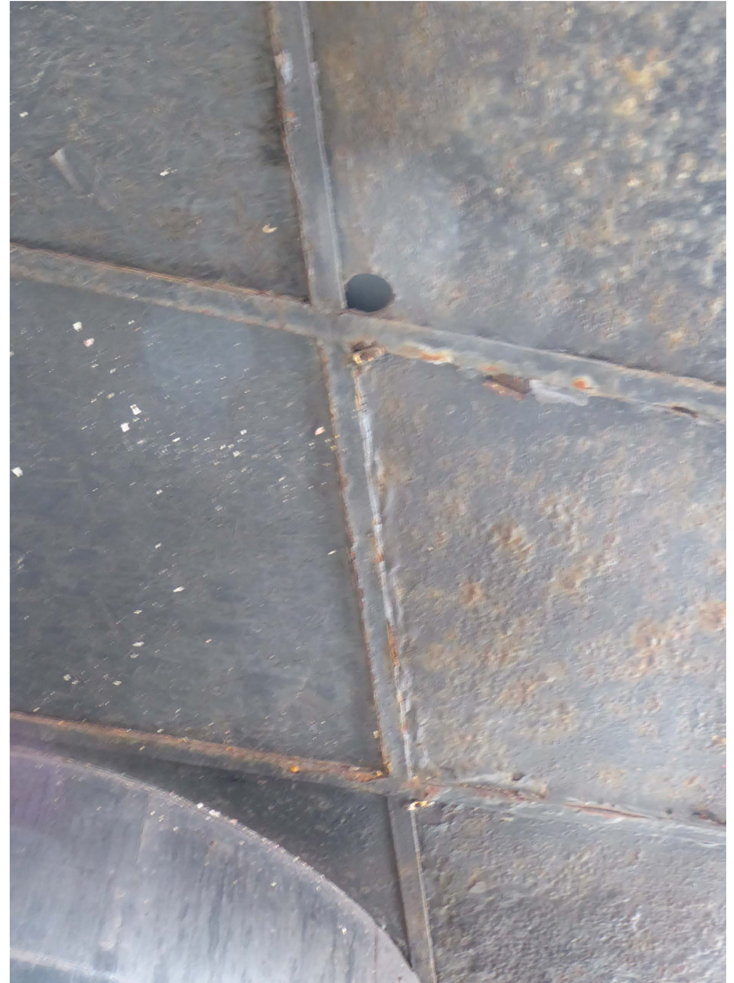
Detailed view of panels and frame
