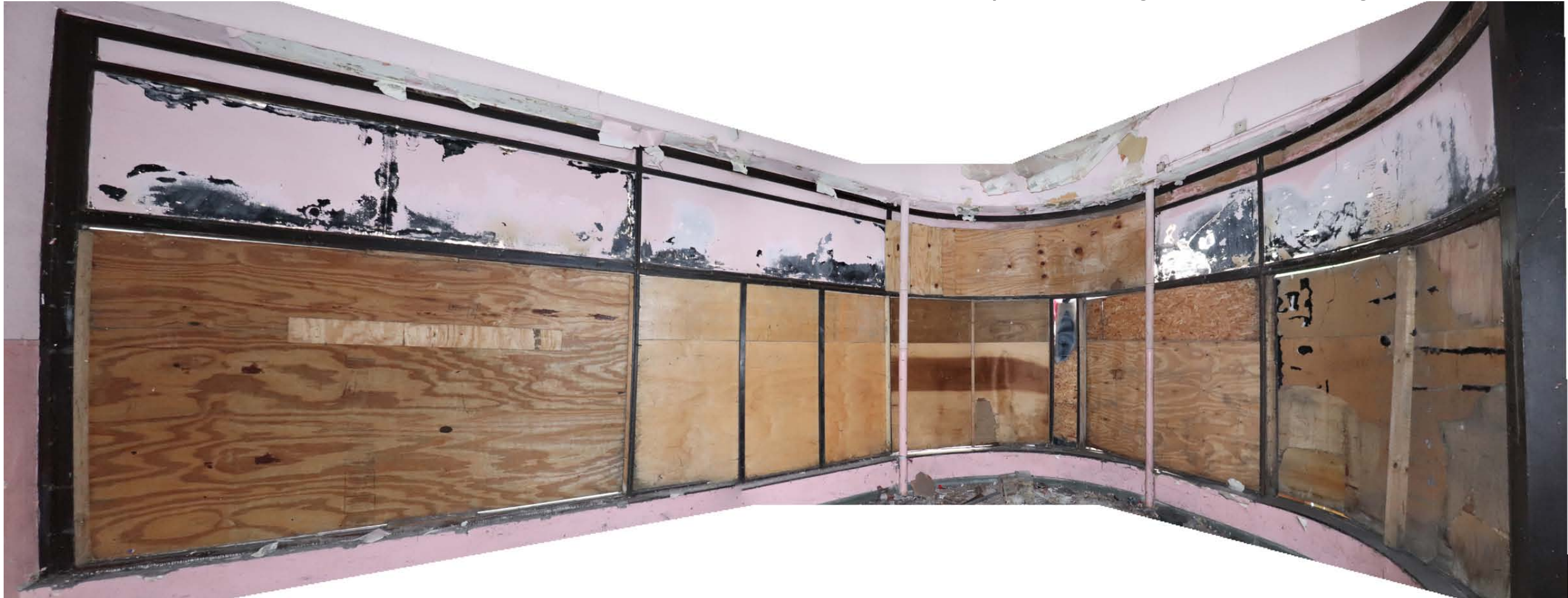
Panoramic View of Glazing with Curved End and two Steel Columns and full extent of boarded up glazing panes
