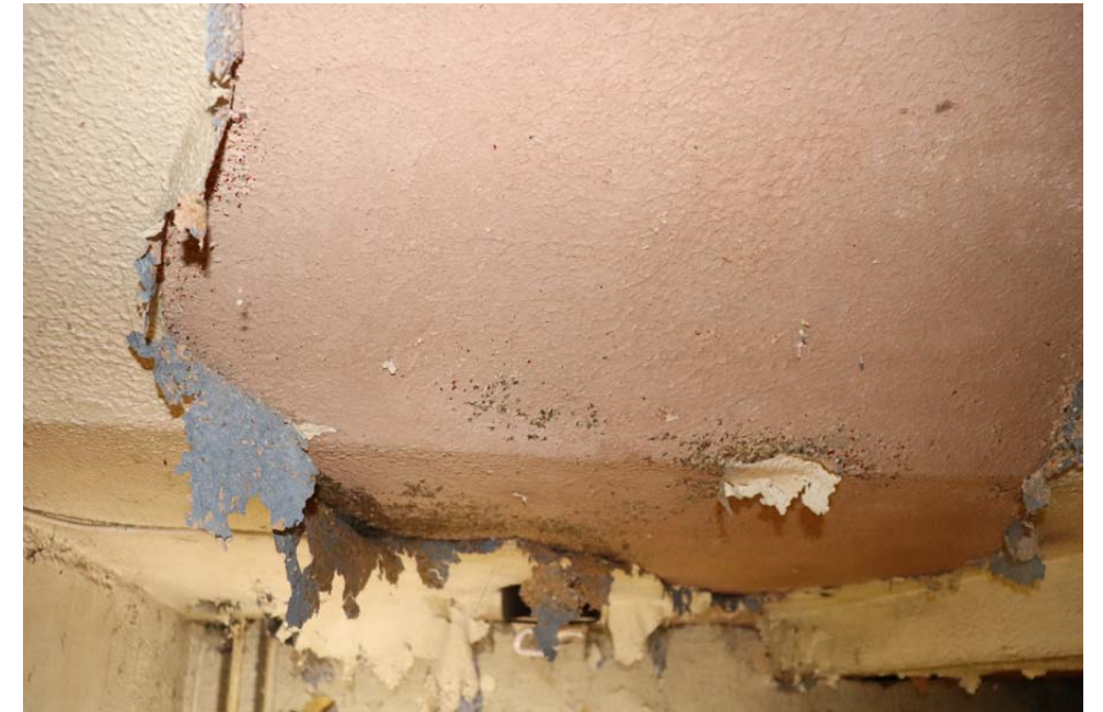
View of peeling paint to soffit over staircase
