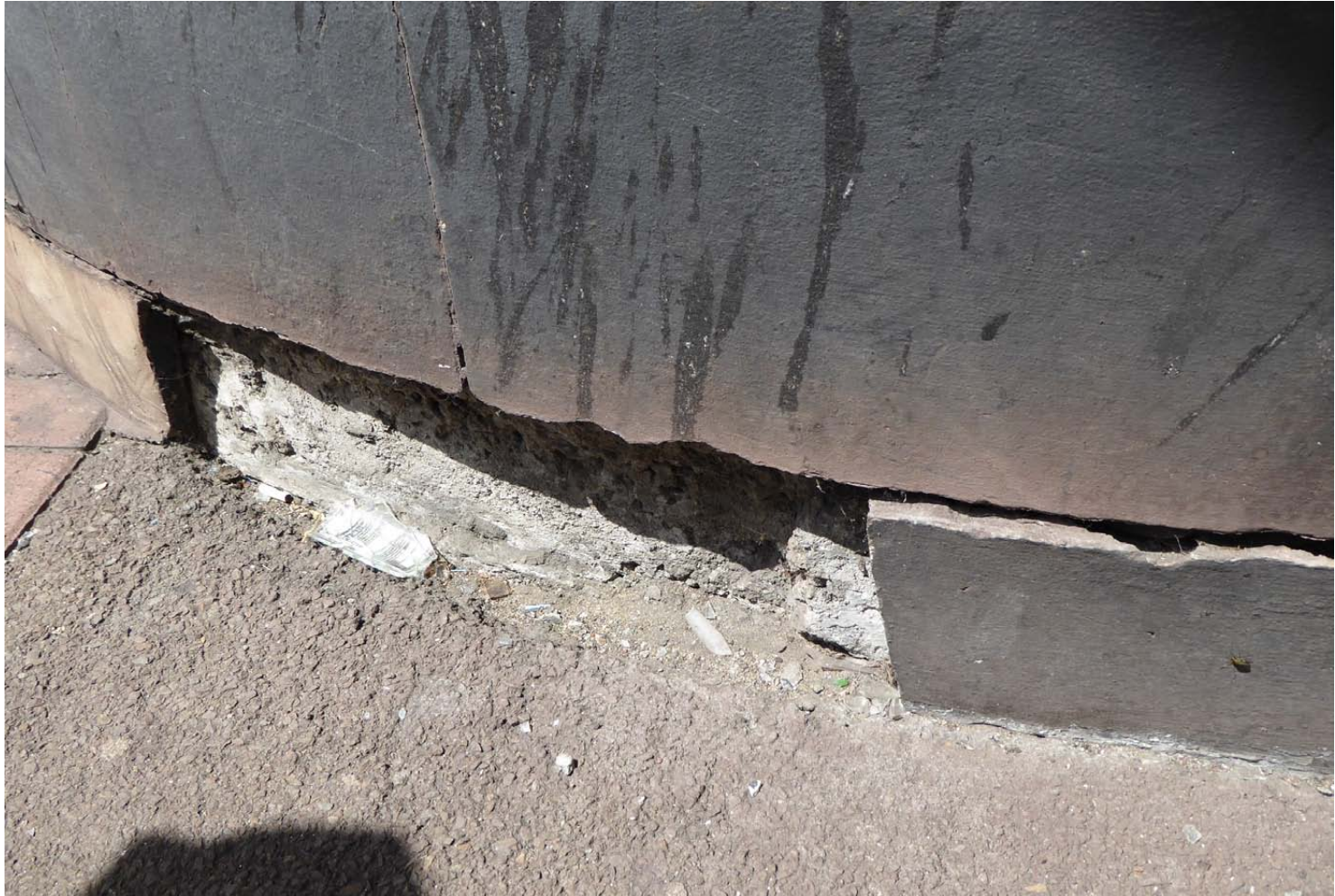
View of spalled surface to plinth
