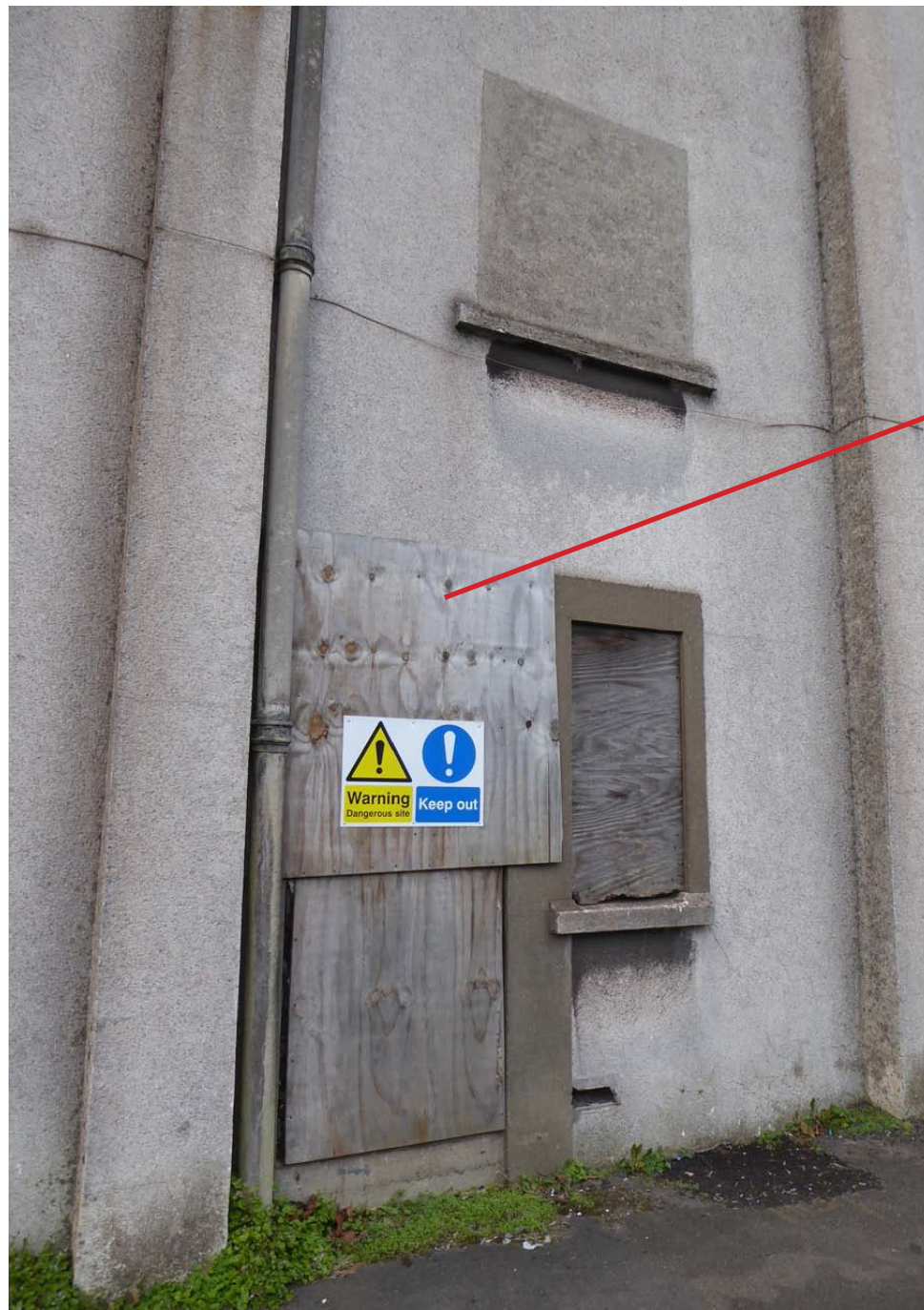
View of blocked / boarded up windows and door to auditorium
