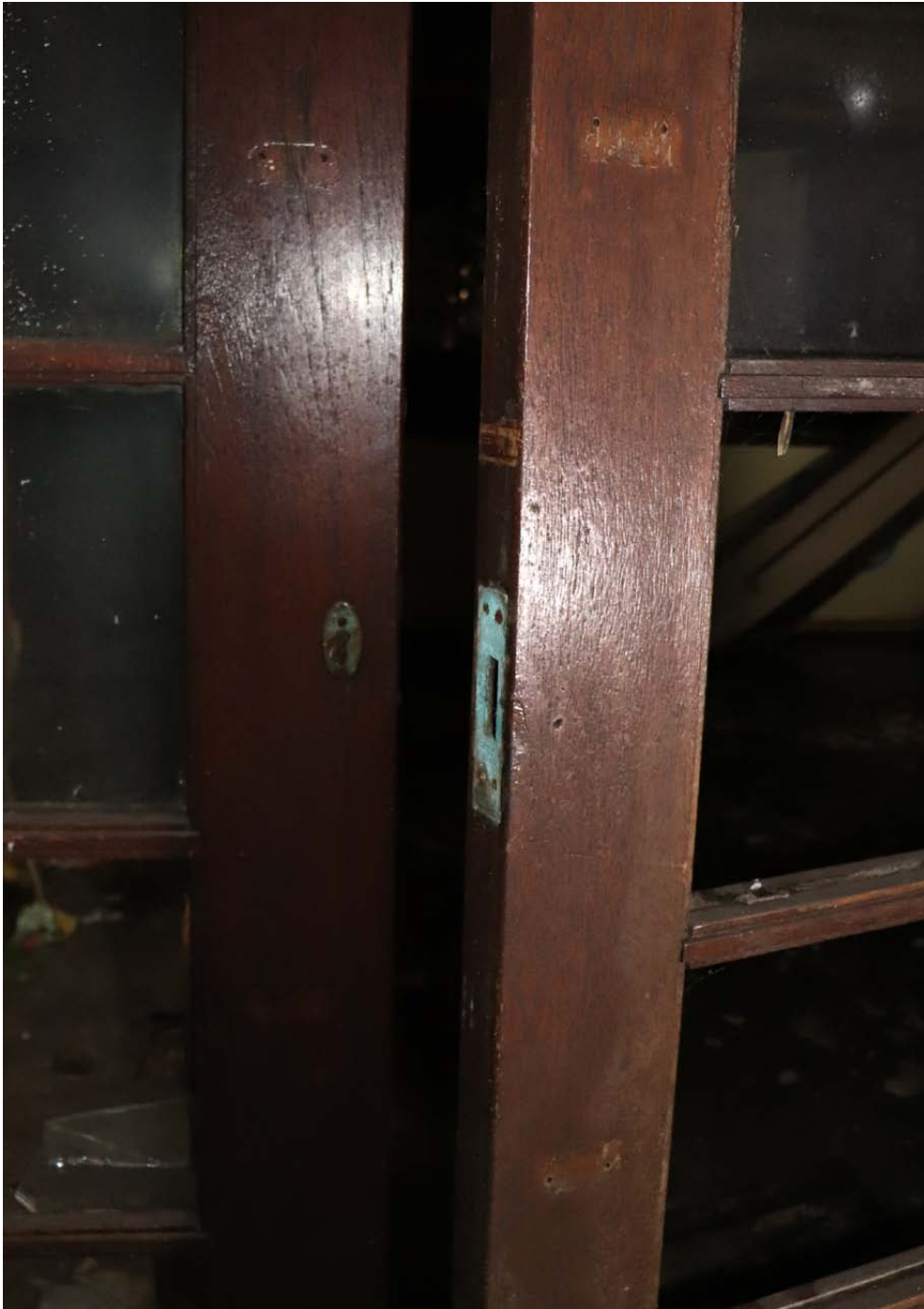
View leading stile of door with holes where handle once was
