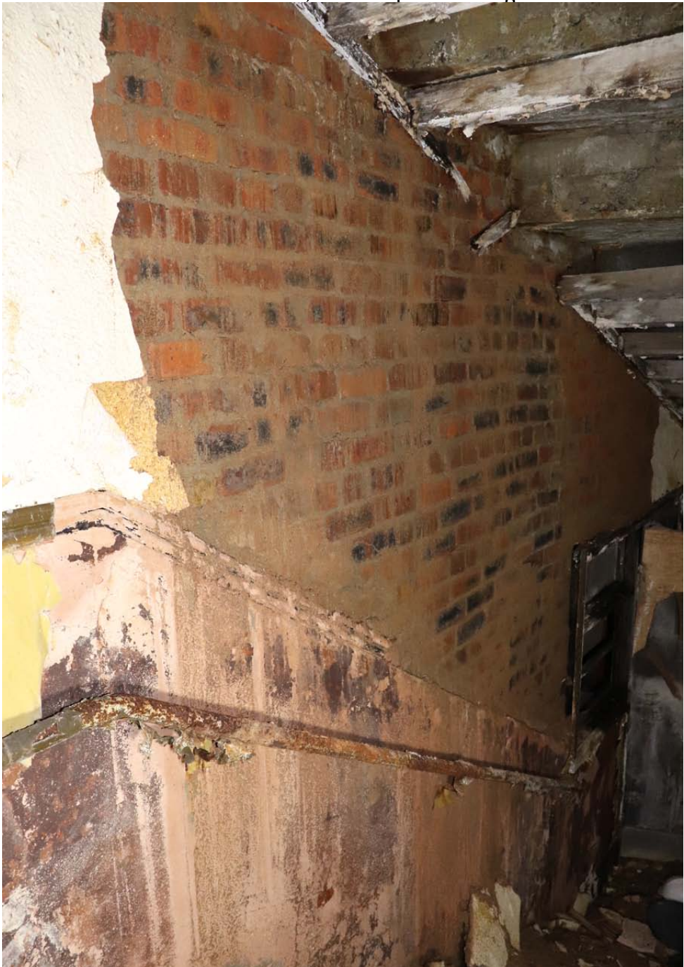
View of saturated brickwork & lost plaster to inner wall
