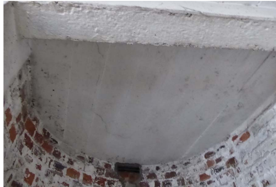
View of concrete 'lid' to turret, showing small crack
