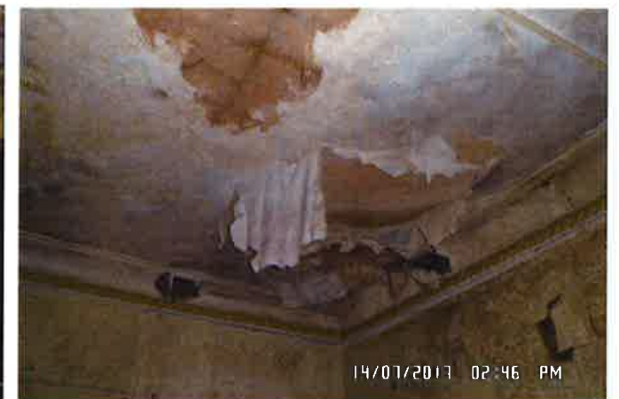
Cracked ceiling slab/damp, July 2017
