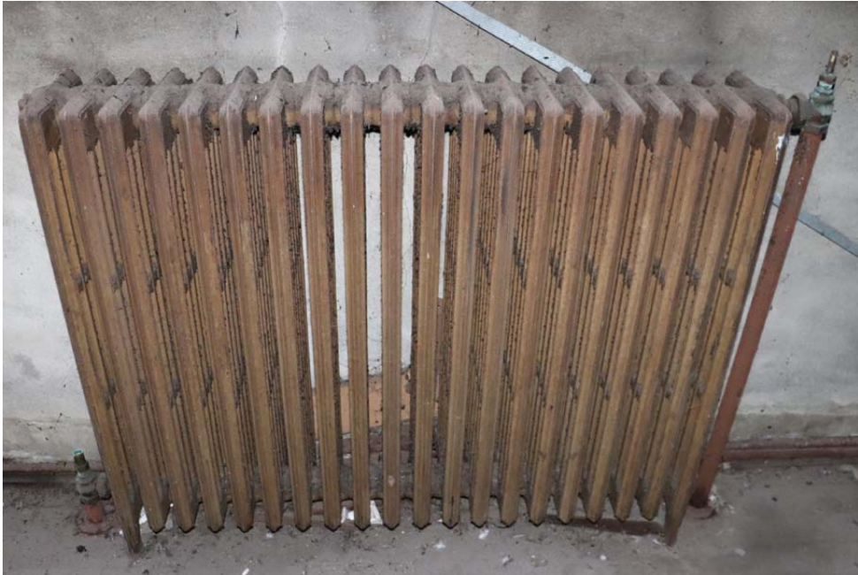
View of cast iron radiator sitting at rear of stage
