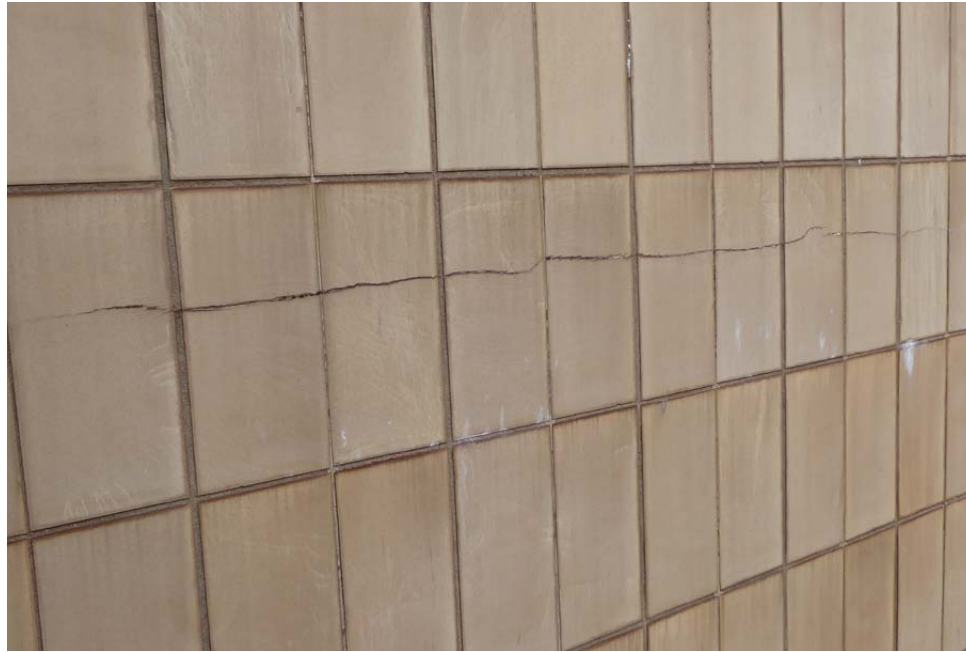
A Cracks in Faience Tiling
