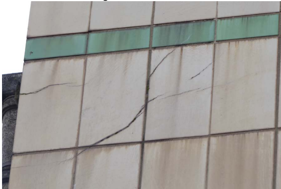
A Cracks in Faience Tiling
