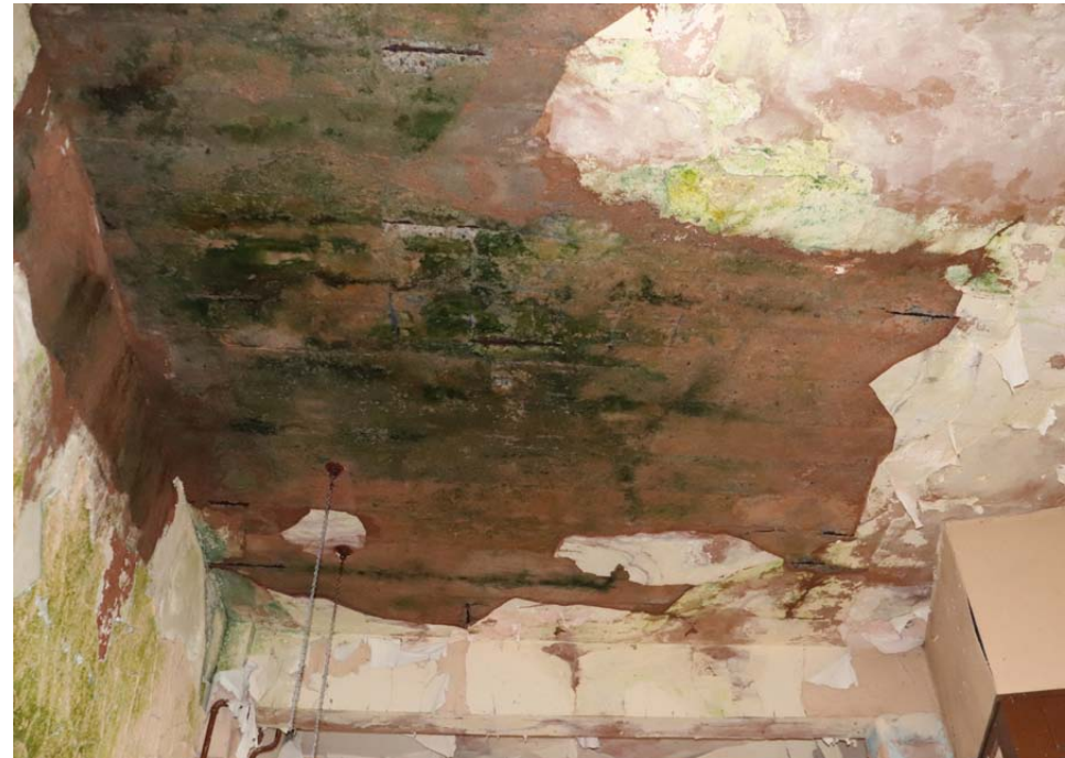
Extremely damp concrete soffit with paint & plaster all lost
