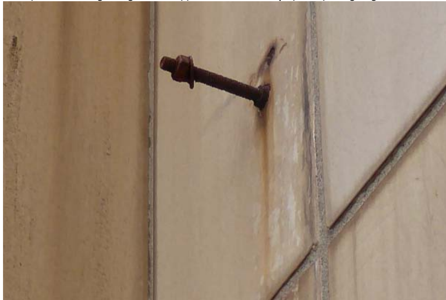
View of a metal fixing in a faience tiling discolouring the tiles
