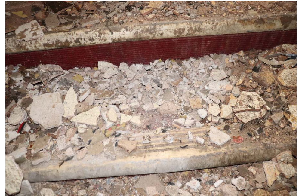
View of carpeted timber stairs with pvc nosings & debris from above
