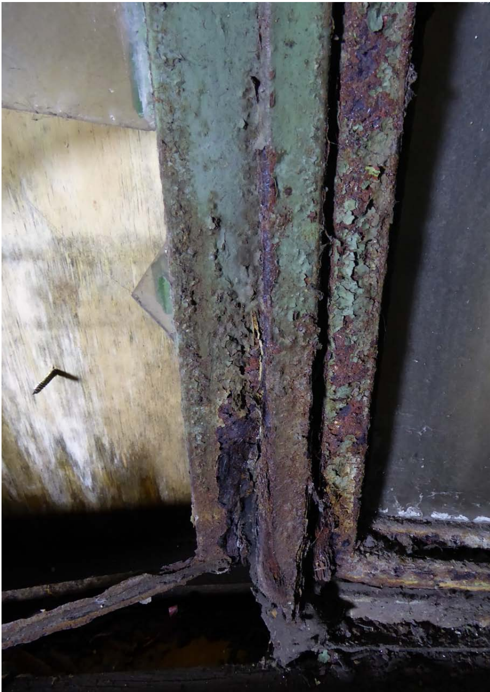
View of the severe corrosion to the steel section at the mullion
