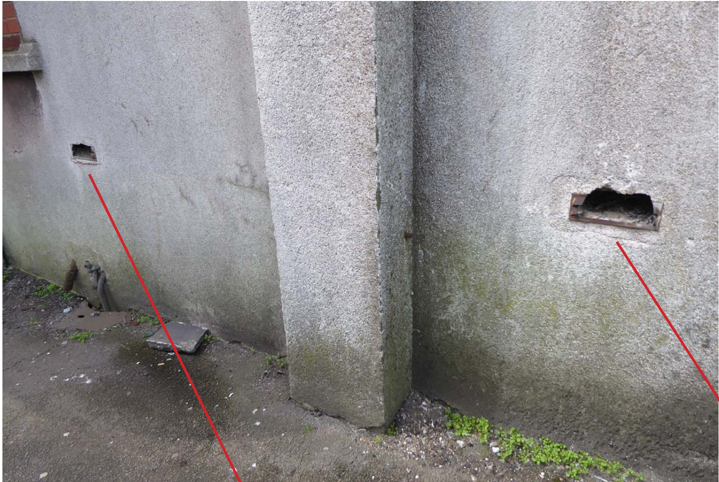
View of two of the broken low vents to the auditorium and cinema
