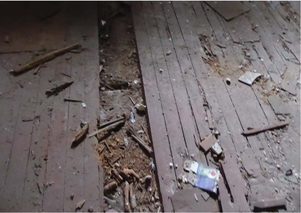
View of timber boarded flooring to auditorium in poor condition
