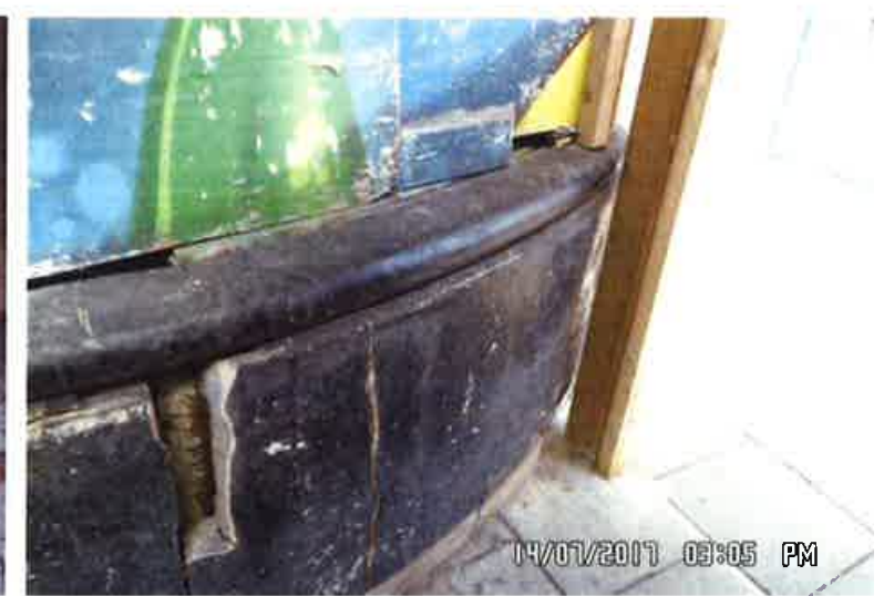
Additional cracking July 2017
