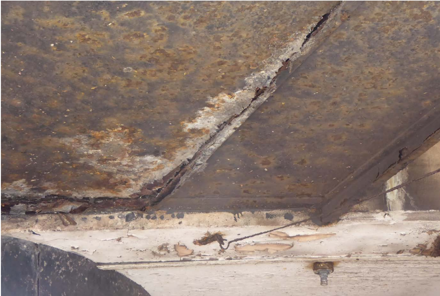
View of two panels abutting each other where 'T' section support appears to have been lost
