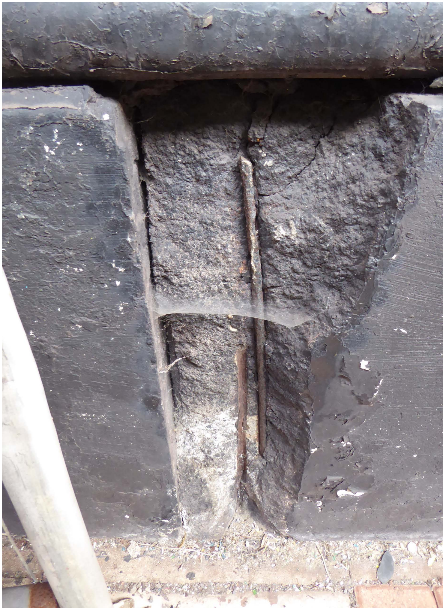
View of spalled surface to plinth showing corroded steel behind which presumably caused the spalling
