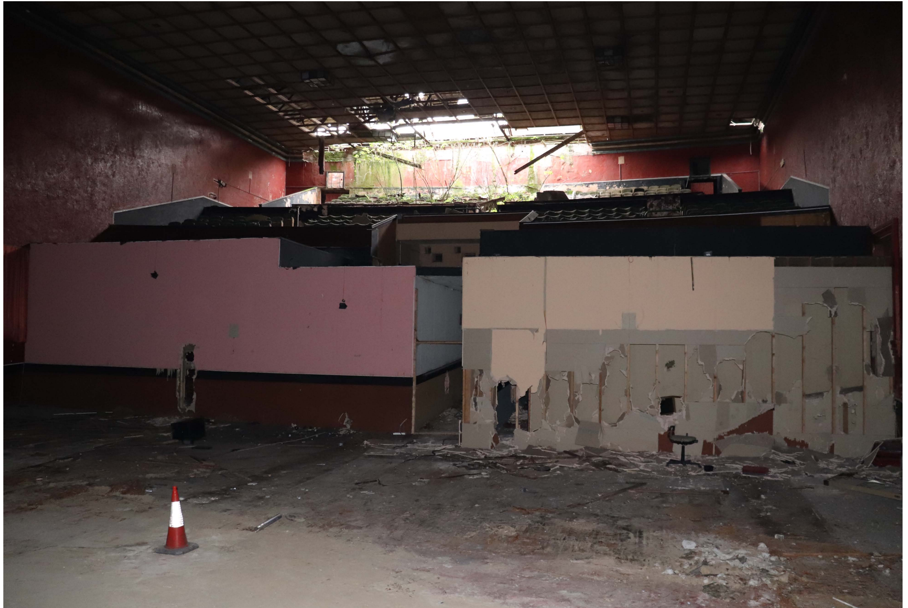
G17 - Auditorium - View looking from stage back to Auditorium, with upper balcony seating and large hole in roof at rear, and plasterboard on timber studwork enclosure to both cinemas with central corridor in between both
