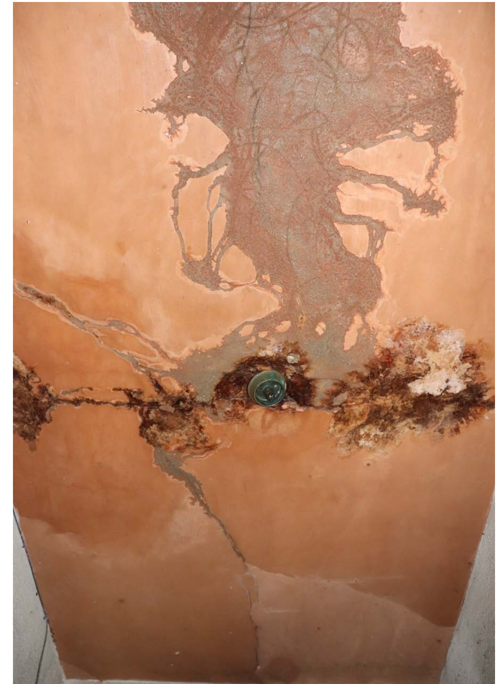
View of ceiling in poor condition
