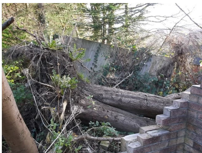
T6 – View of stems fallen through boundary fence
