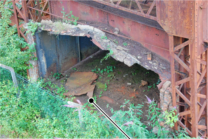
HEADFRAME 1: Accumulation of debris over plates to be removed. Fallen metalwork from within ventilation shaft to be retrieved for inspection.
