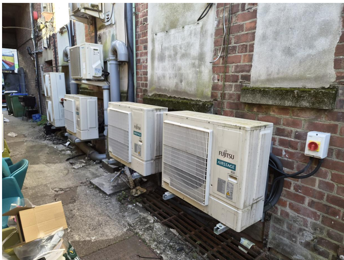
FIGURE 2: INSTALLED PLANT INCLUDING 3X APPLICATION UNITS
