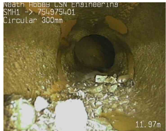
2, 00:01:02, 11.97 m Settled deposits, fine, 10% cross-sectional area loss
