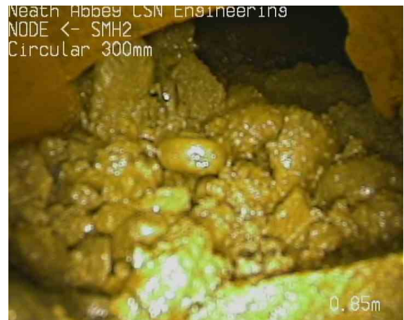
2, 00:00:23, 0.85 m Collapsed drain or sewer, 50% cross-sectional area loss
