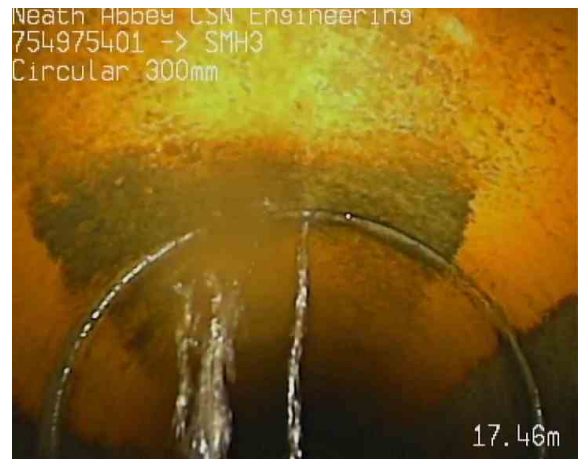
2, 00:01:38, 17.46 m Infiltration, gushing from 11 o'clock to 12 o'clock
